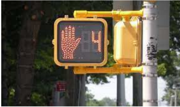
Figure 7-10 Example of a VRU Countdown Timer (Source: Chicago Metropolitan Agency for Planning)
