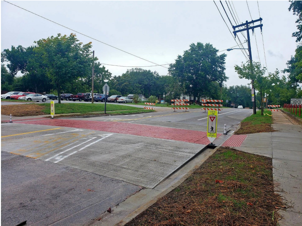
Figure 7-4 Example of a Raised Crosswalk Installation in Springfield (Source: CivicEngage, 2022)
