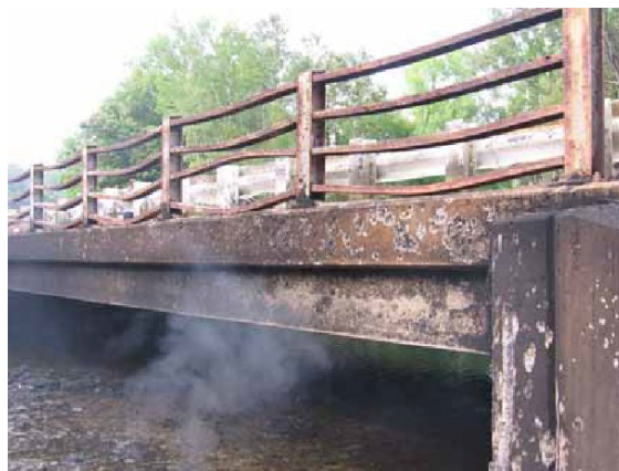
Figure 52 Fire damage (Graybeal 2007)
