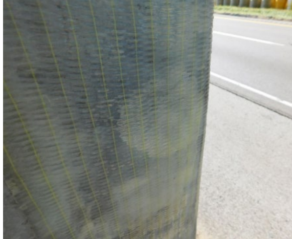
Figure 45 Potential void (Baniya et al. 2022)
