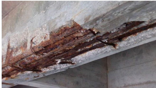
Figure 26 Corrosion in steel reinforcement embedded in concrete substrate (Jung, Jeong, and Lee 2022)
