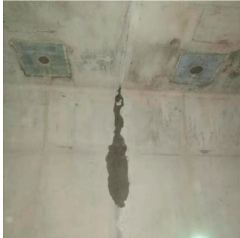
Figure 50 Water seepage (Wang and Fan 2020)
