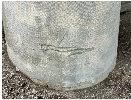
Figure 12 Scratch caused at the externally applied FRP (Source: FHWA)
