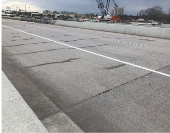
Figure 28 Top surface cracks in GFRP reinforced bridge deck (Shafei 2023)
