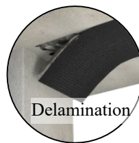
E.3 Concrete Delamination
