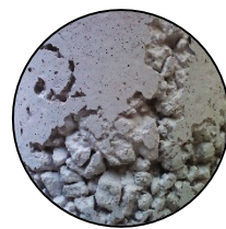
E.2 Concrete Voids
