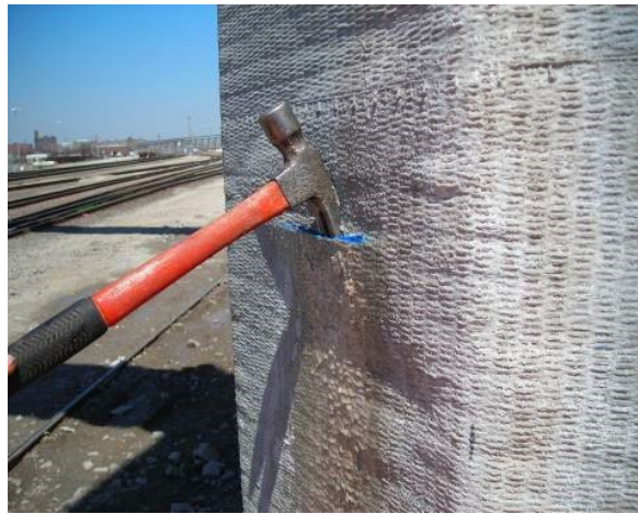
Figure 39 Rupture due to moisture entrapment (Source: Authors)
