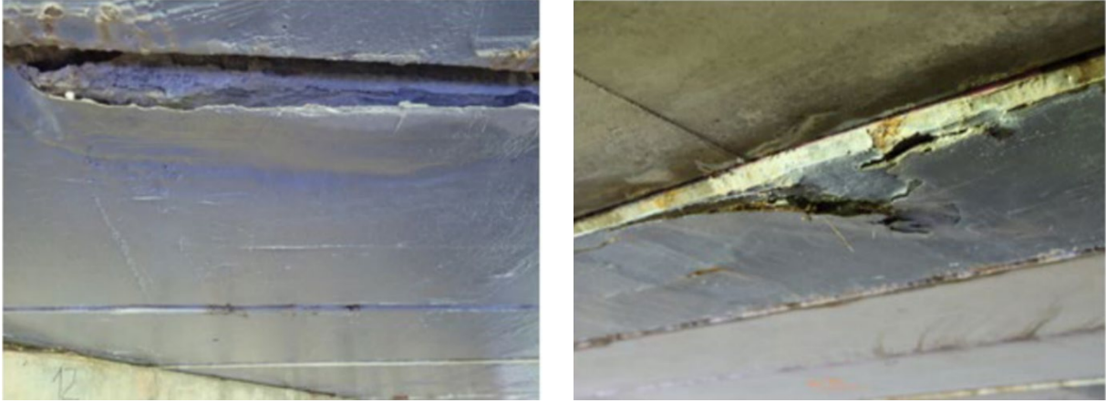
Figure 46 Spalling of substrate concrete causing tearing of externally applied CFRP (Baniya et al. 2022)
