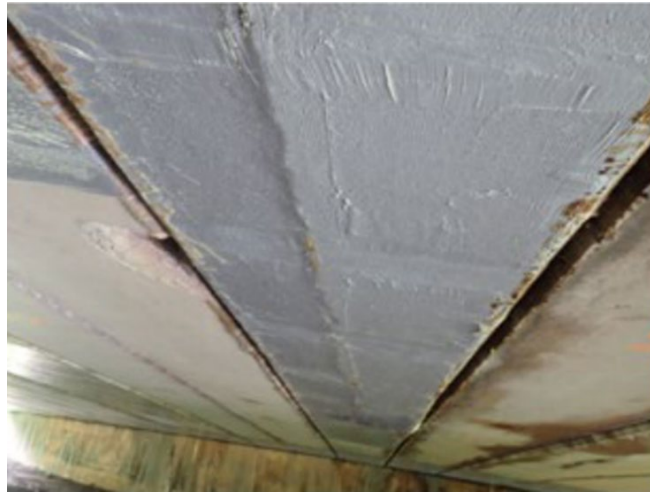
Figure 47 Bulged CFRP layer indicating the presence of a longitudinal crack beneath (Baniya et al. 2022)
