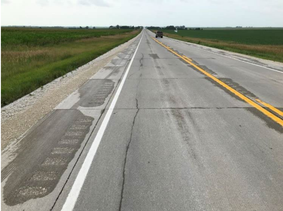
Lots of longitudinal cracking.
