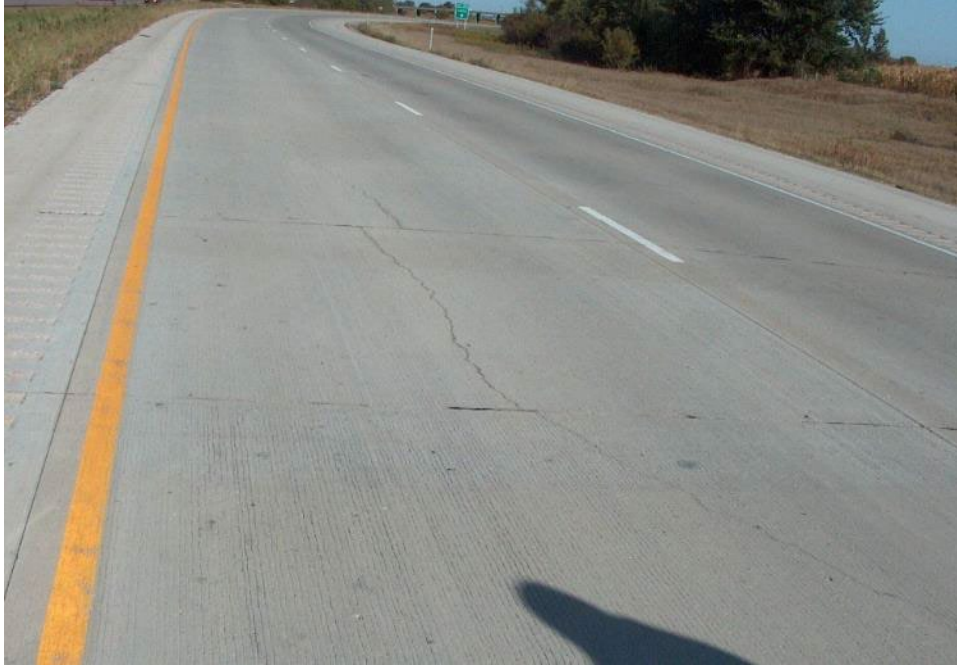
Figure 49 – Woodbury I-29 NB Longitudinal Cracking – passing lanes.
