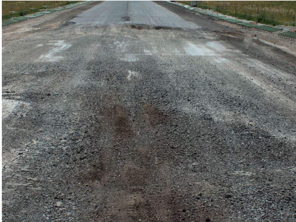
Figure 32 – HMA deterioration on US 71 Cass Whitetopping Project
