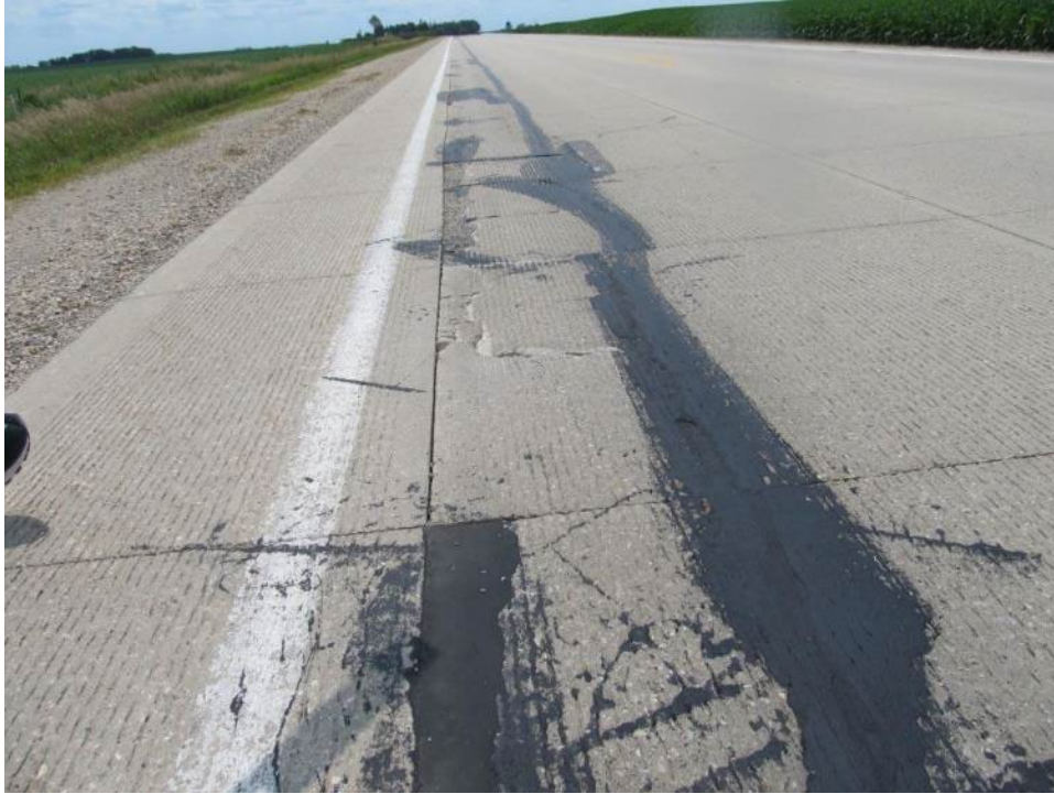
Figure 21 – Grundy IA 14 Longitudinal Cracking and Shattered Panels
