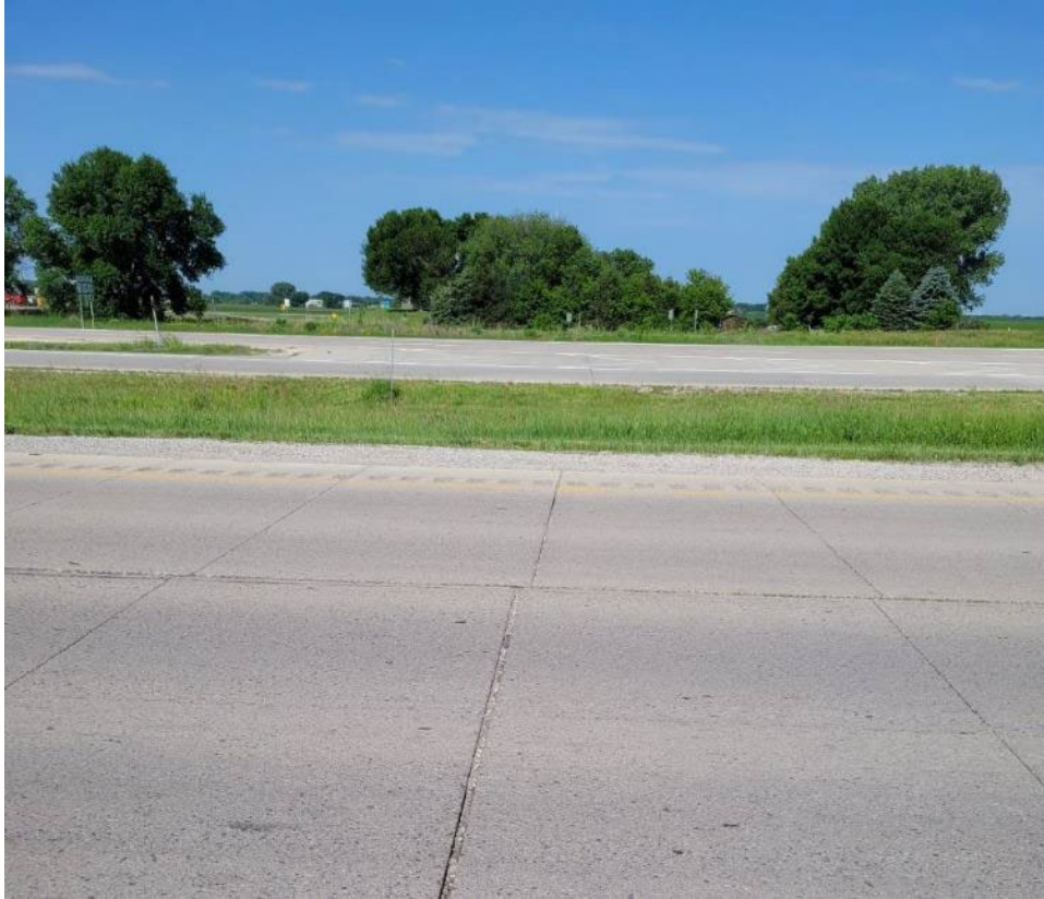
Figure 33 – Clay/Dickinson US 71 NB panels migrating in driving lane at BOP against HMA pavement.
