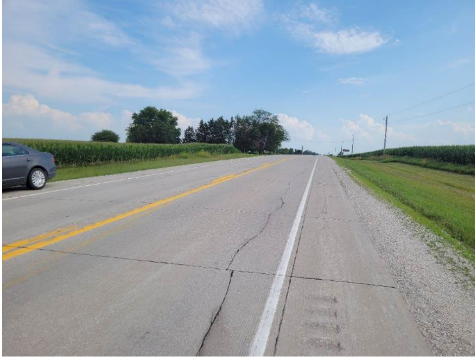
Figure 22 – Dallas US 169 UBOL Longitudinal Cracking
