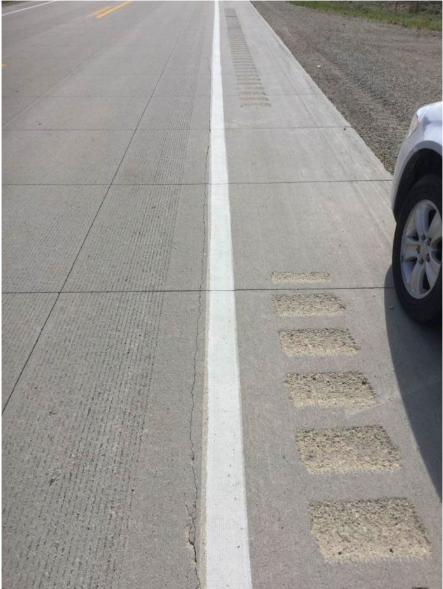
2017 – Cracking at 4 ft from edge. Location of old edge of widened pavement.
