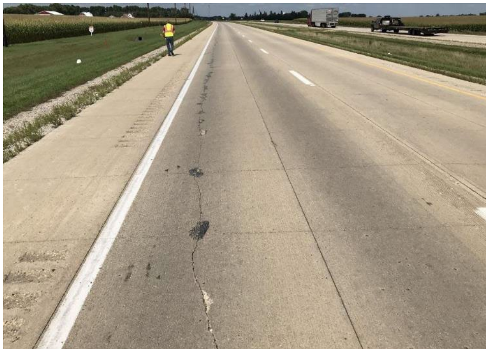
Figure 39 – Typical cracking off end of steel in wheel path.
