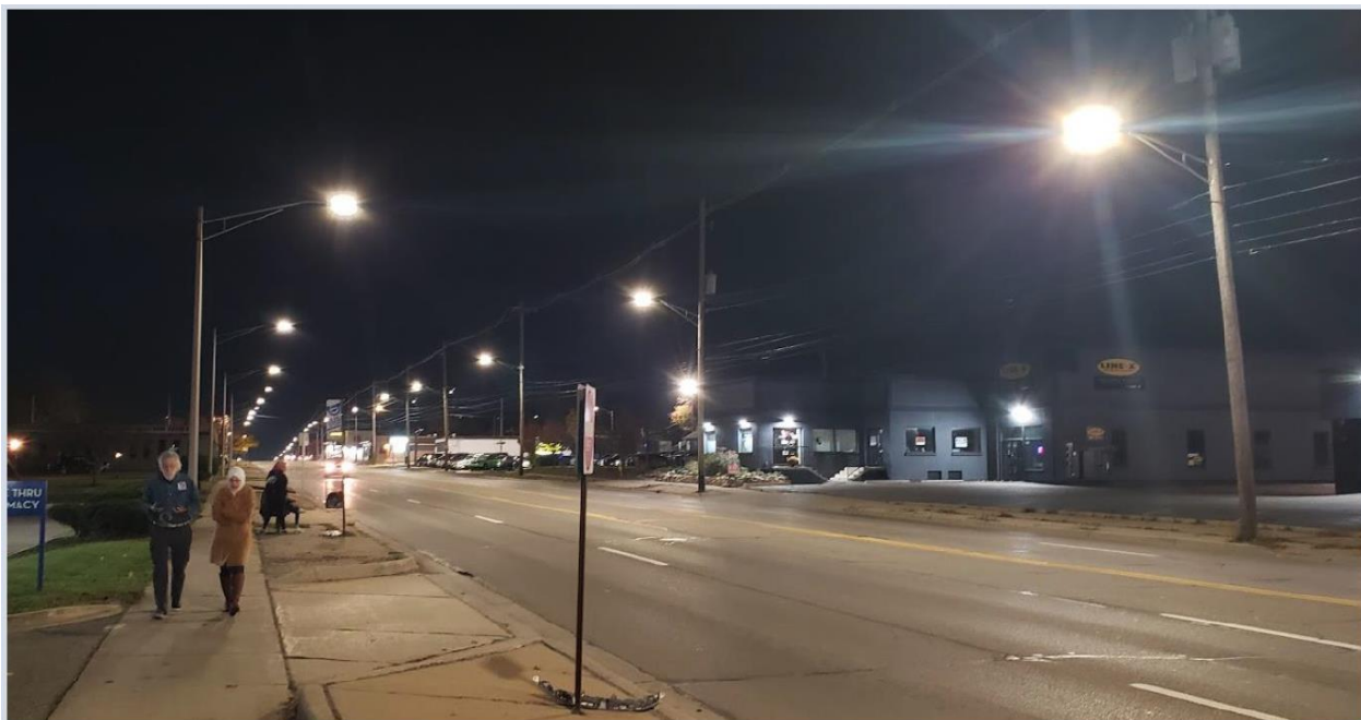
Figure 4-18. Lighting condition along S. Cedar St., Lansing
