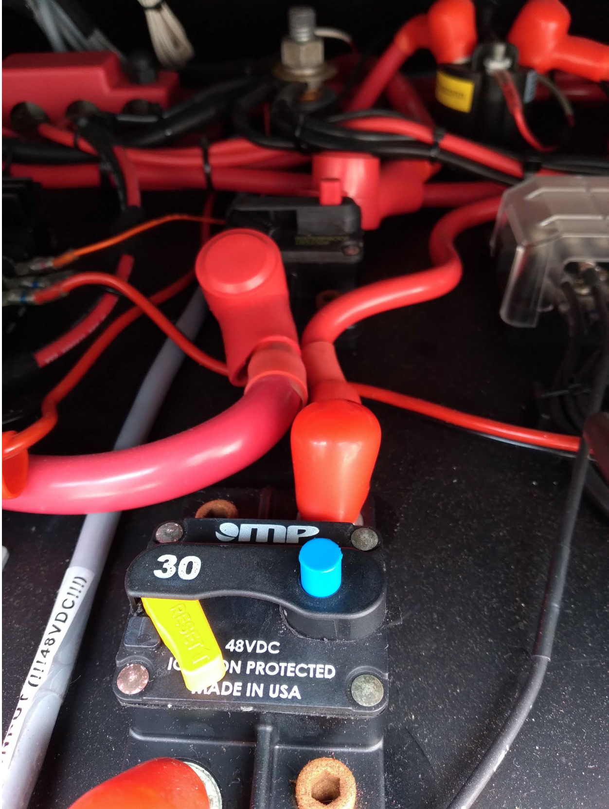
Image 4: 2 breakers underneath on bottom shelf in cabinet
