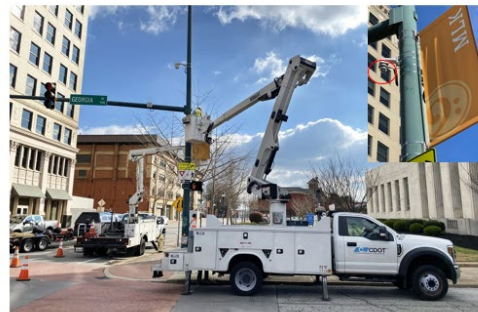
Figure 3. Photos and text. Current roadside or infrastructure-based LiDAR ITS applications in Nevada and Tennessee [22].
