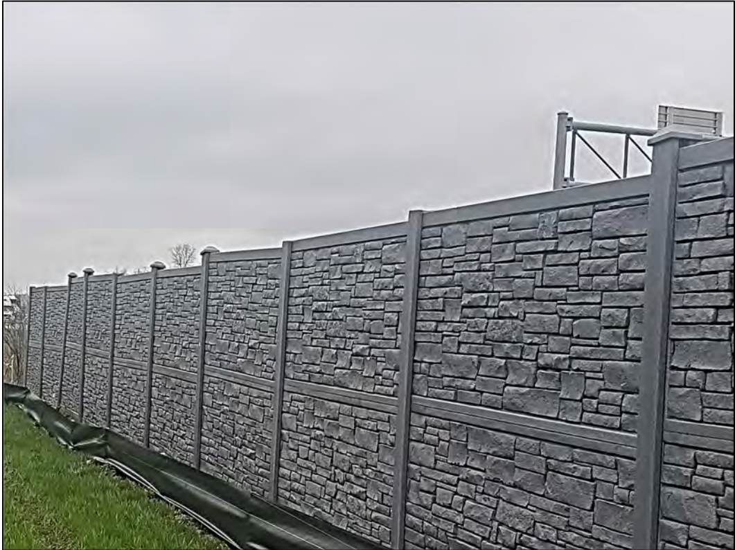
(14) Wall lines not parallel and missing post caps
