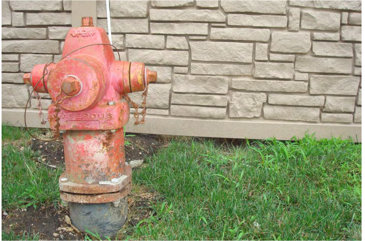
Gap at the bottom of one of the panels. In front of this panel was a fire hydrant.
