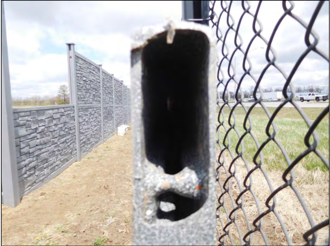
(03) Missing upper reinforcement beam in damaged panel
