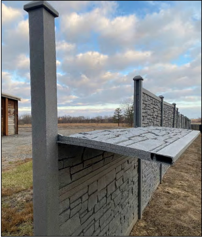
(01) Broken panel on the south side of the wall
