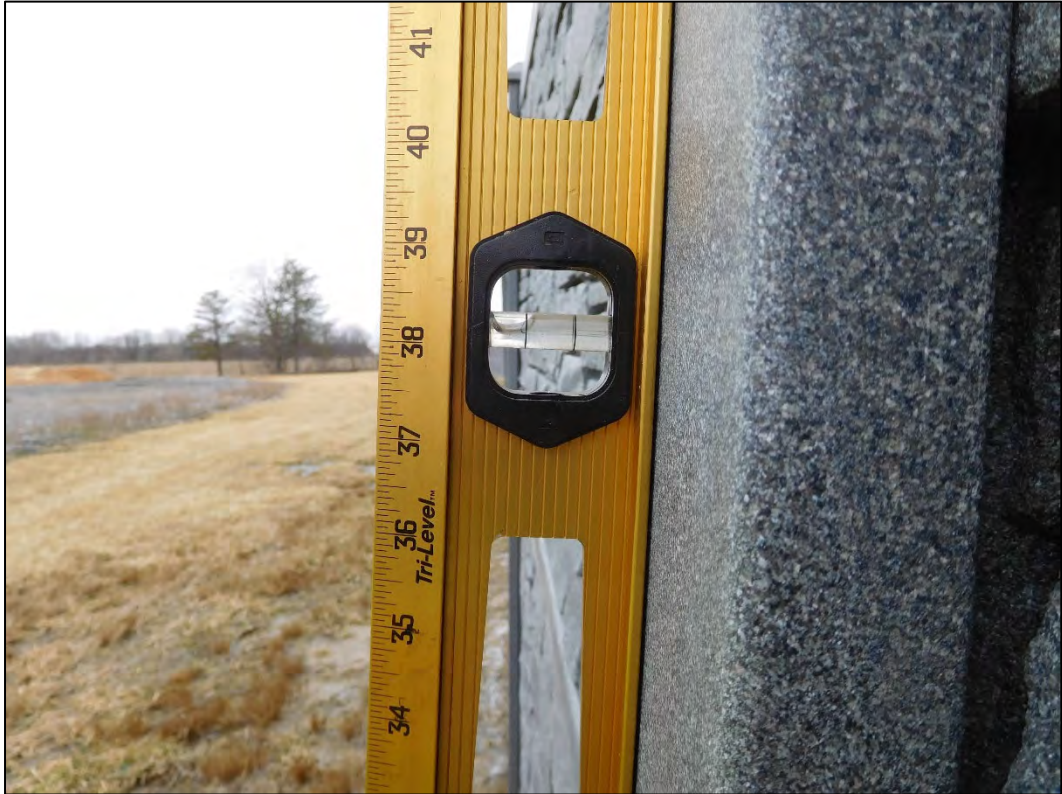
(02) Posts out of vertical plumb shown by the bubble level
