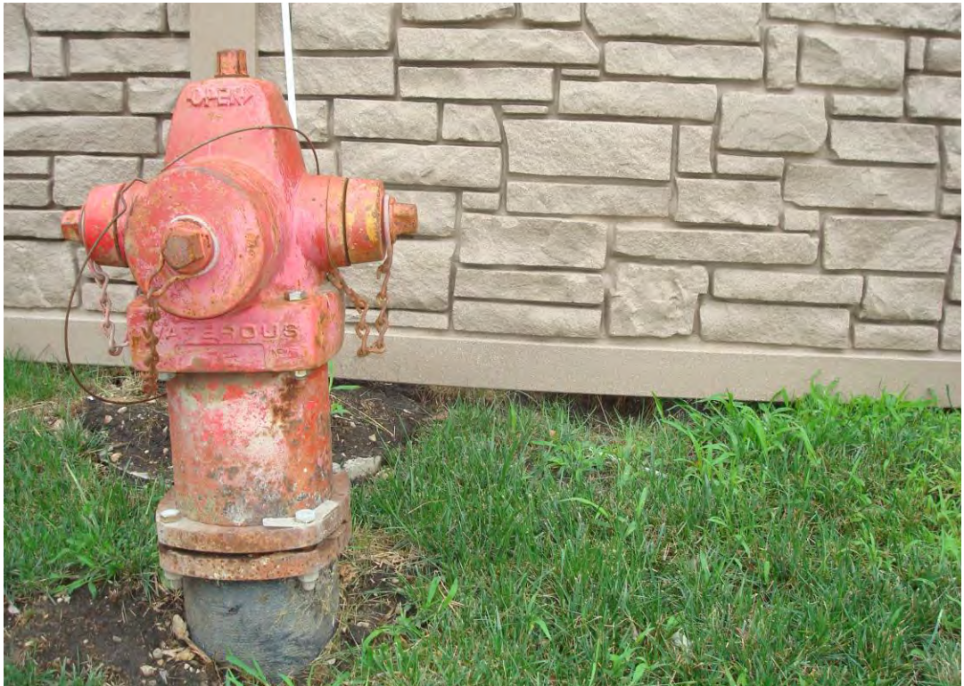
(7) Gap at the bottom
