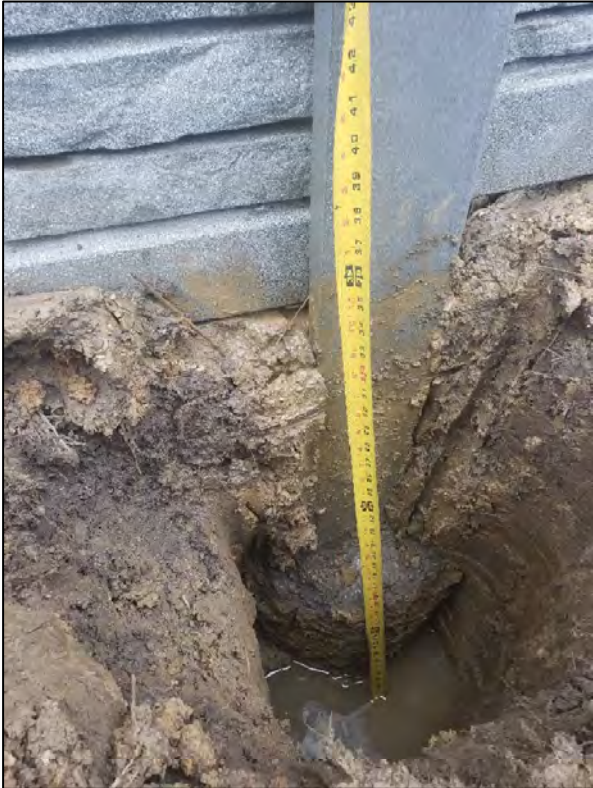
(28) Post 5 ponding of water below top of concrete footer
