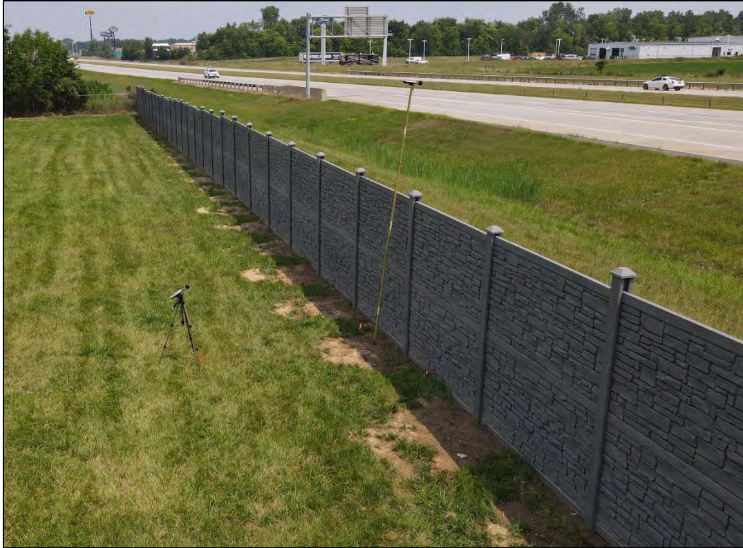
(11) Drone aerial image of Meter A and B in Lima, OH after vinyl wall construction
