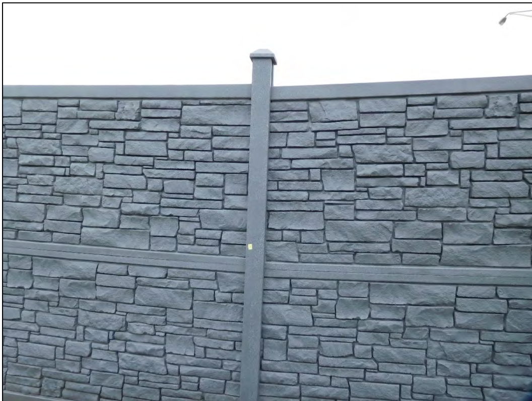
(10) Settling of post/panel
