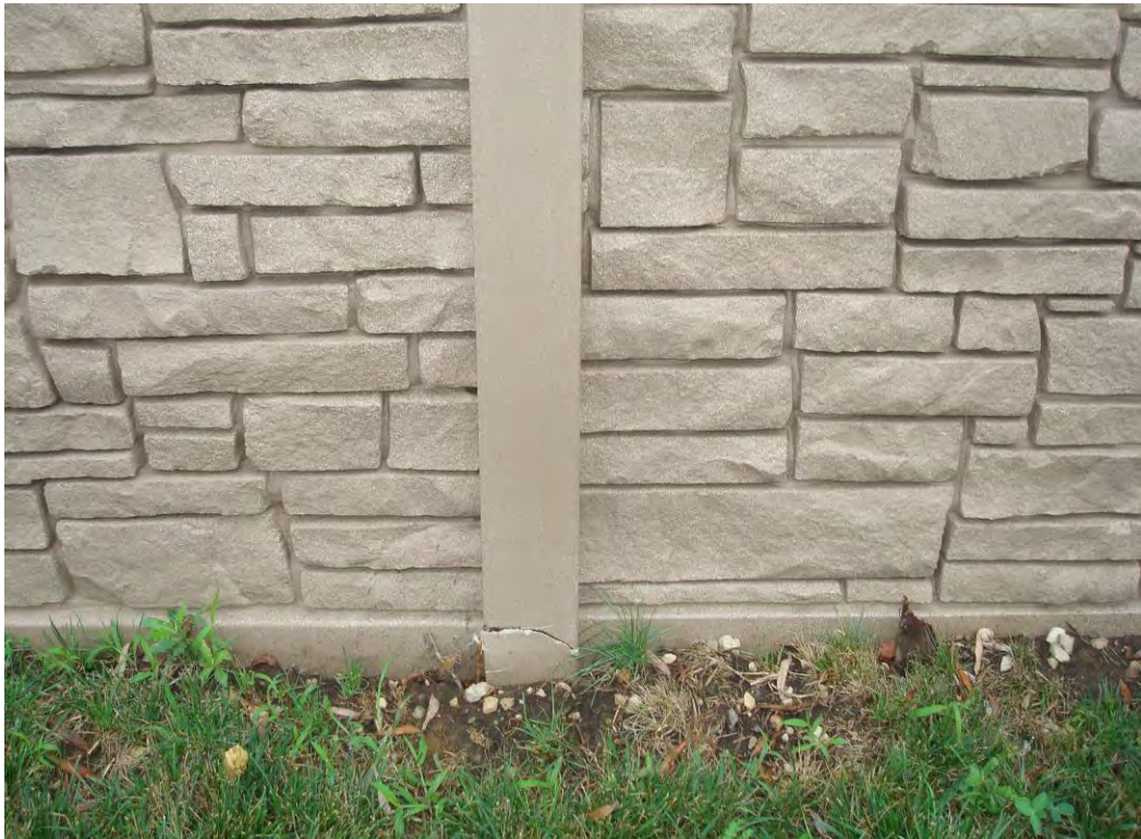
(5) Crack at bottom of one of the posts.
