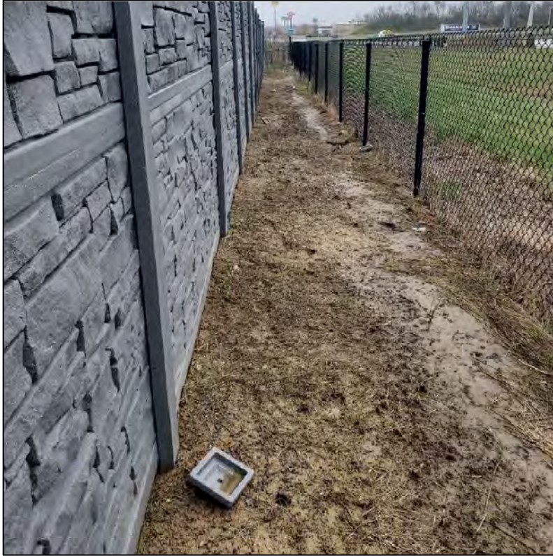
(15) Post caps fallen to the ground
