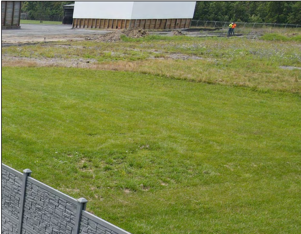
(13) Meter E (beside crew members) in Lima, OH after vinyl wall construction
