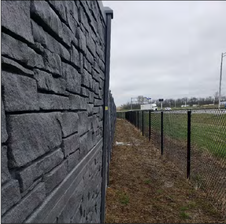
(09) Post 4 out of vertical plumb
