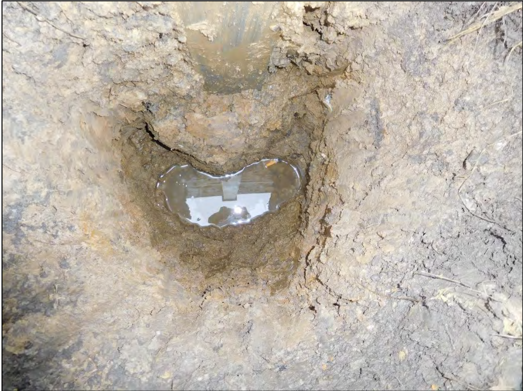
(26) Post 4 ponding of water below top of concrete footer
