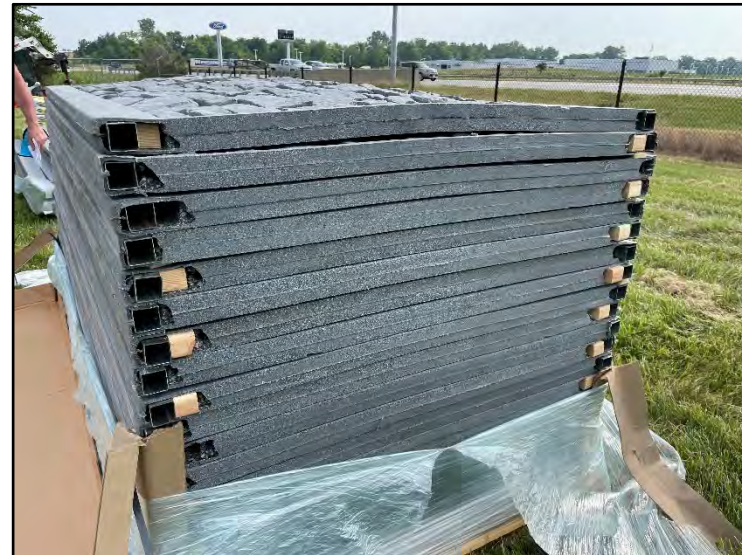
(06) Wooden blocks under steel reinforcement, purpose unclear
