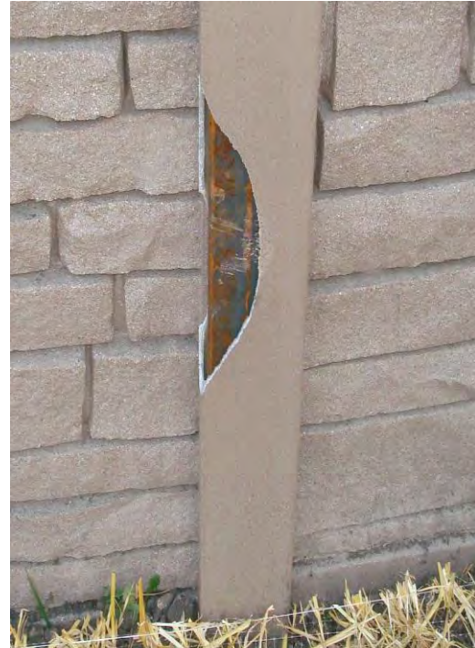
Figure9 a vinyl post is broken
