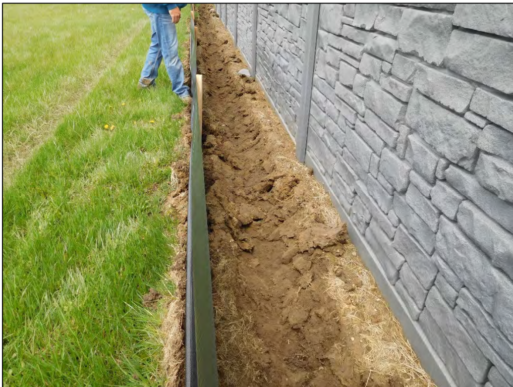
(20) Depth of depression in the soft ground adjacent to the wall made by a lightweight tractor used to install the silt fence
