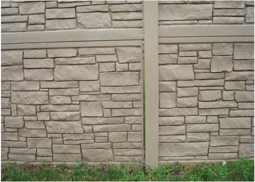
(6) Gap on between one of the panels and the post
