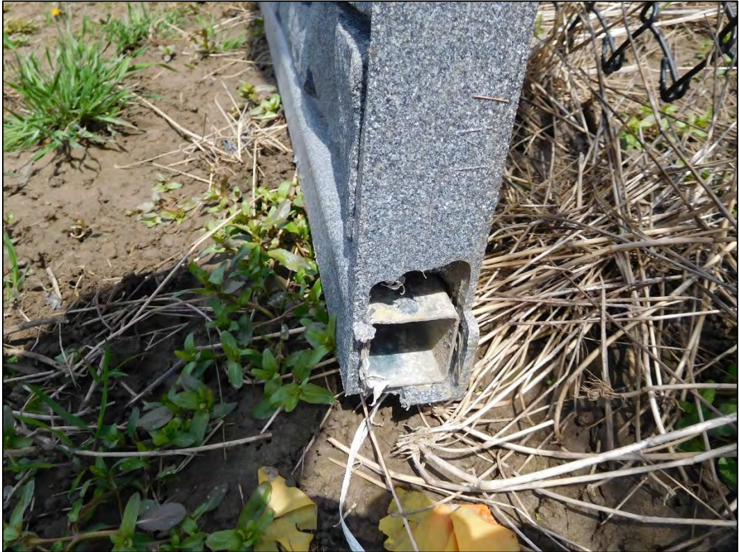
(04) Bottom of damaged panel with reinforcement beam in place
