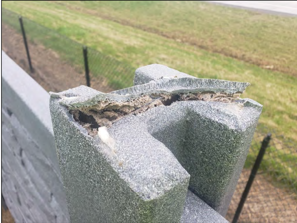
(17) Top of the post damaged
