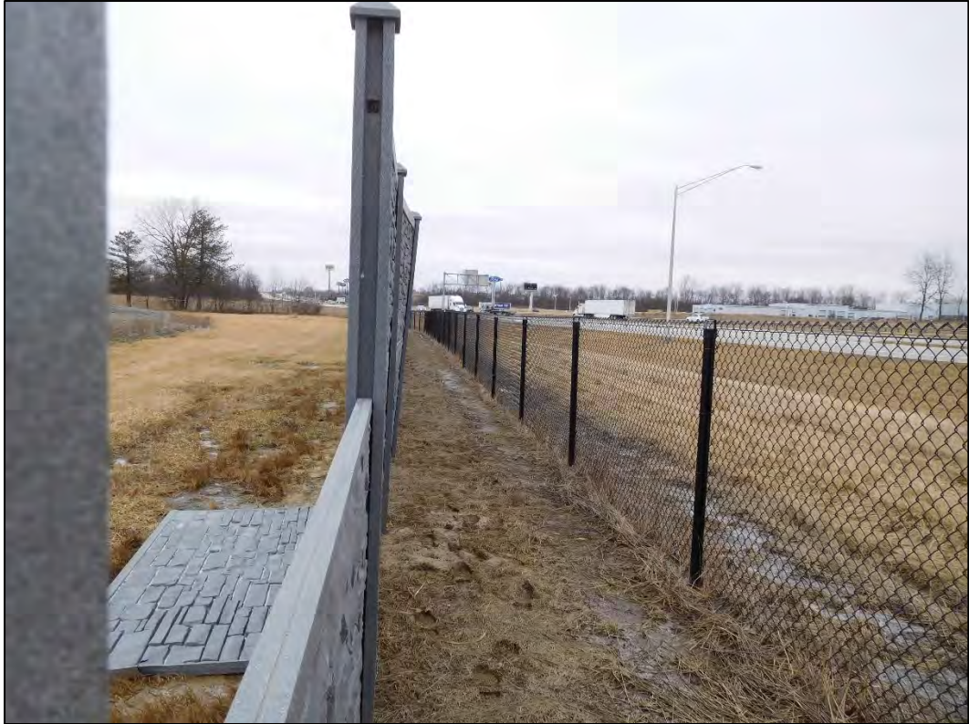
(01) Posts visibly out of vertical plumb
