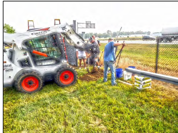
(12) Clearing of dirt from drilled hole. 4 cubic-feet of concrete went into each posthole.
