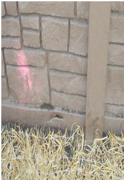
Figure8 crack at the bottom
