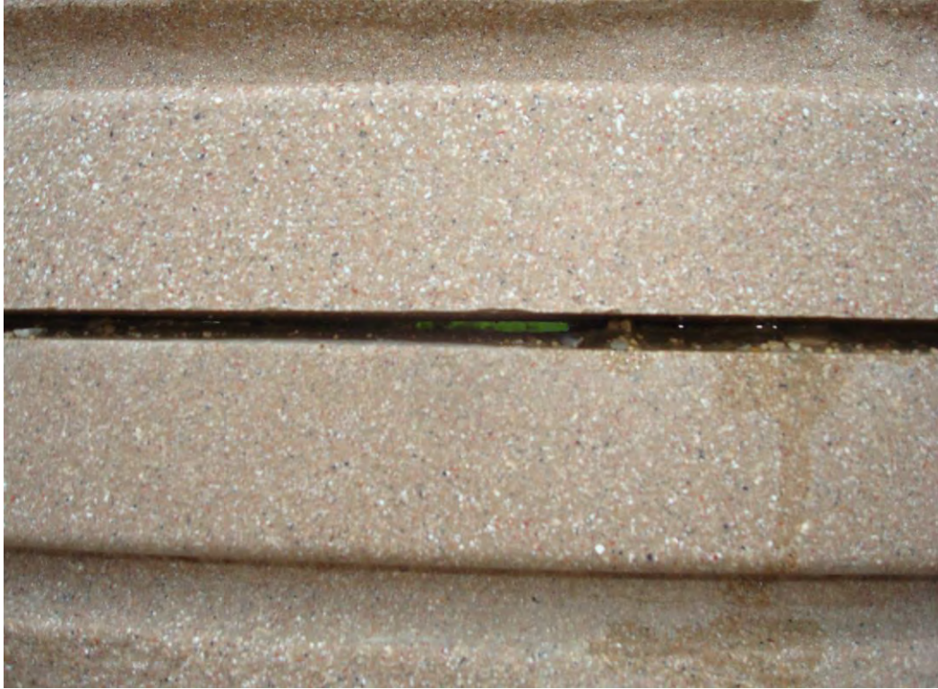
(4) Westside south gap between two of the panels.
