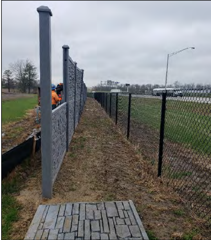
(01) View of the broken panel
