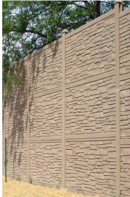
Figure5. (12 feet Vinyl noise wall)
