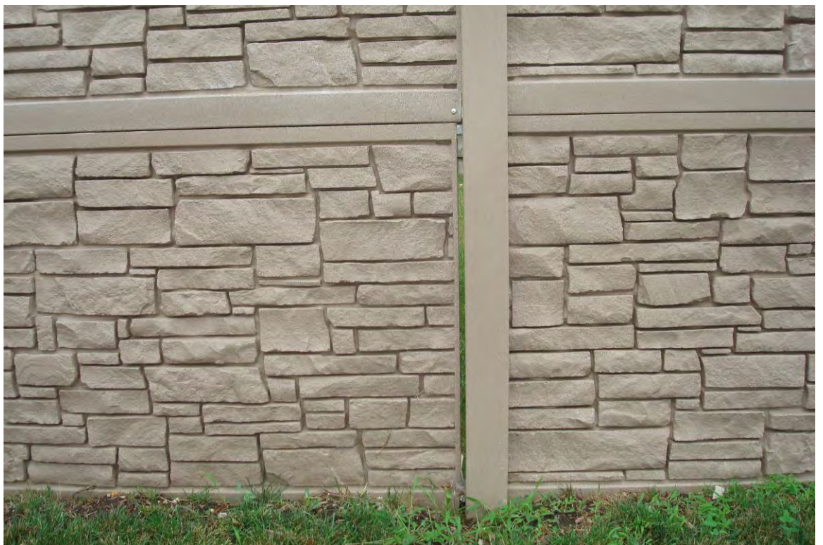
Opening and major gap on between one of the panels and the post
