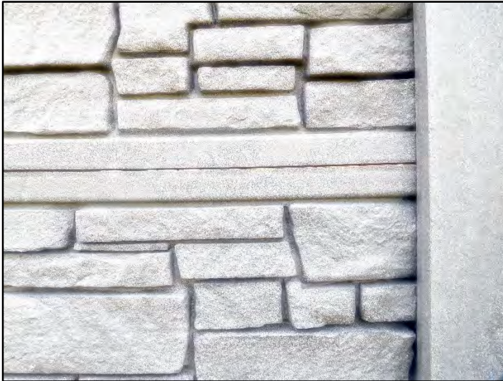
(19) Slight gap between some top and bottom panels due to burrs from form
