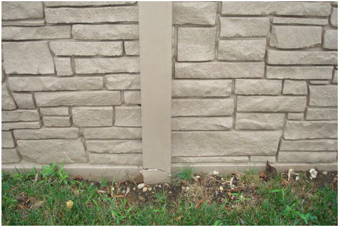
Crack at bottom of one of the posts.
