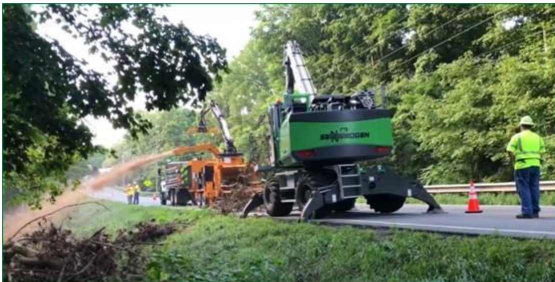
Photo 7: Sennebogen 718E and remote-controlled Bandit 2090 working in tandem moving piles of debris
