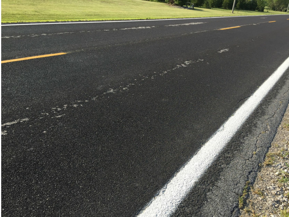
Figure 1. Chip Seal with Slag Section on State Route 66 in Defiance County (Photograph Taken in July 2023, Approximately Five Years after Construction).
