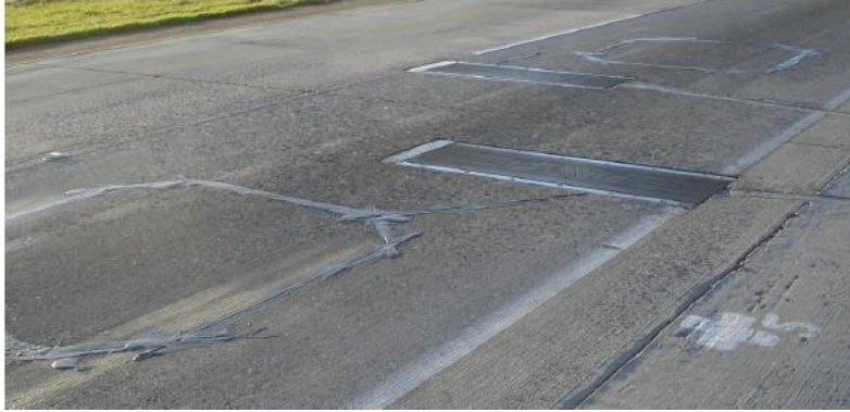
(a) Staggered Bending Plate Installation and Inductive Loops ( Hallenbeck and Weinblatt 2004 )
