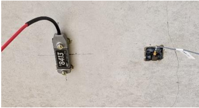
(a) Strain Gauge and Accelerometer at Bridge Ends
