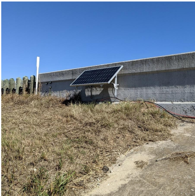
Figure 5.35. Installed Solar Panel (Bridge #3).
