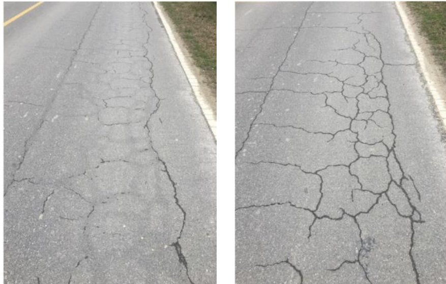
A.1 Pavements with low to moderate crack density.
