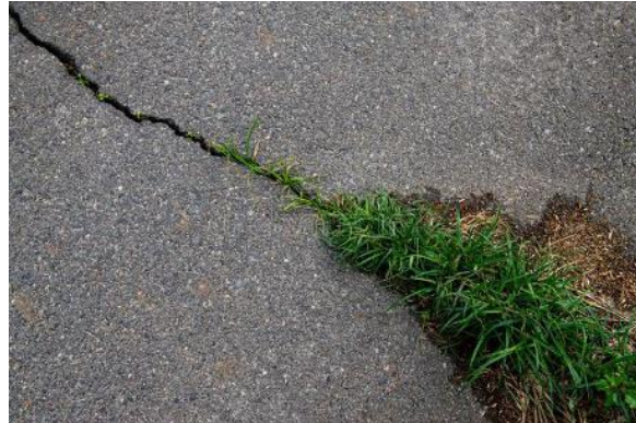
A.3 Pavement crack vegetation.
