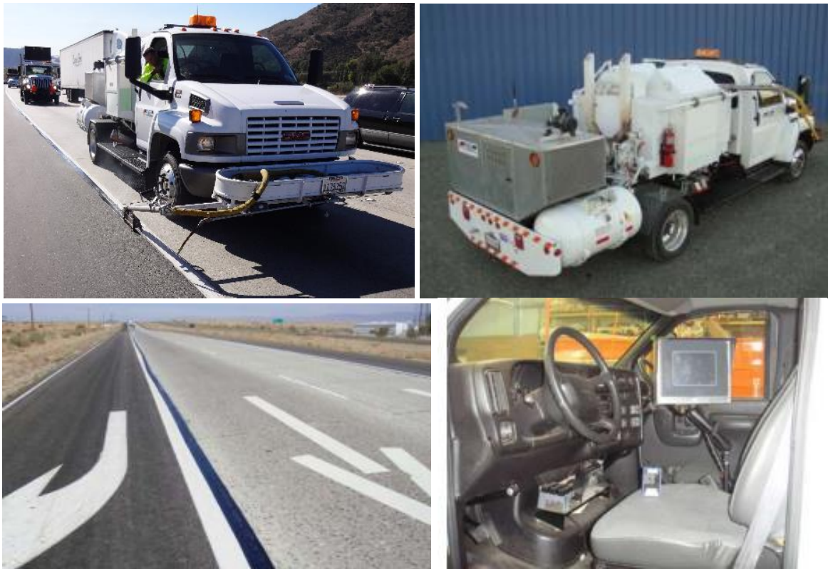
A.7 Sealzall System developed by (AHMCT) (22)
