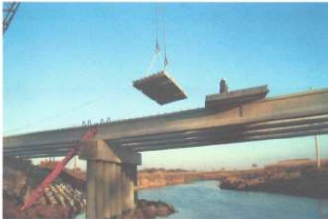
Guided by NCHRP research, the Iowa DOT saves time and money by using prefabricated bridge components.
