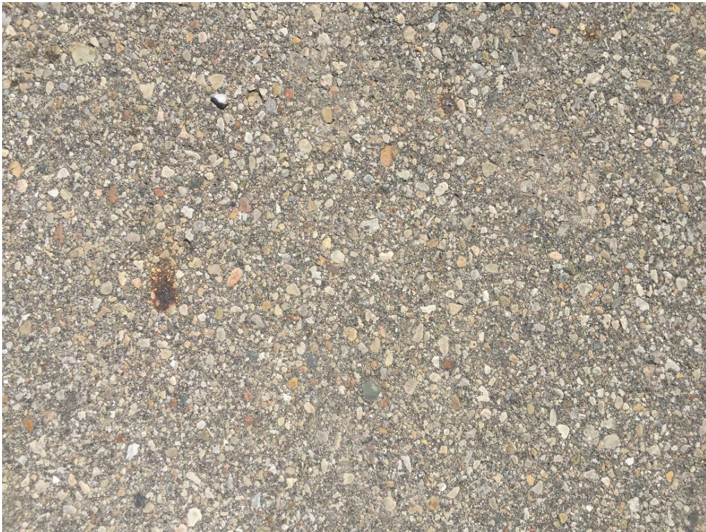
Figure E.5. Photo Taken at Studenbaker Rd. (Last Paved in 2015).
