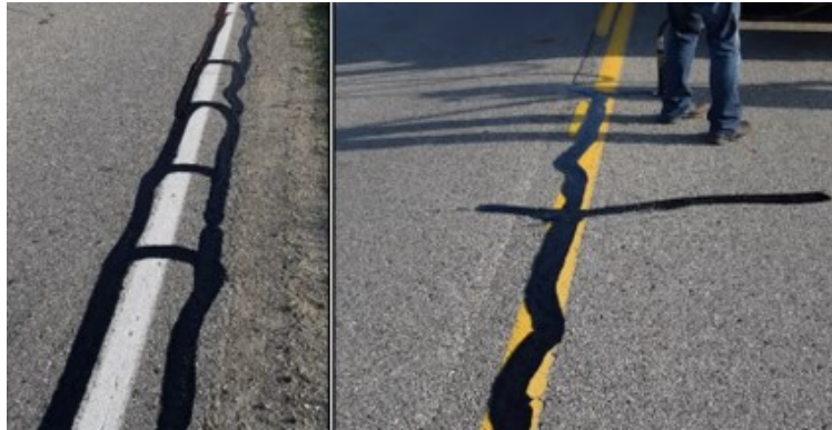
Figure 2.18 Overbanding in Michigan (67)
