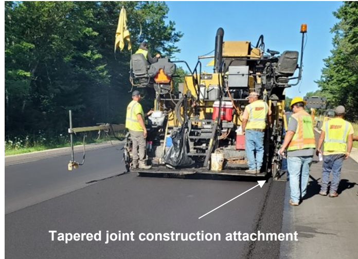
Figure 5.2 Using an attachment for constructing a tapered unconfined joint at the M-28 project, MI
