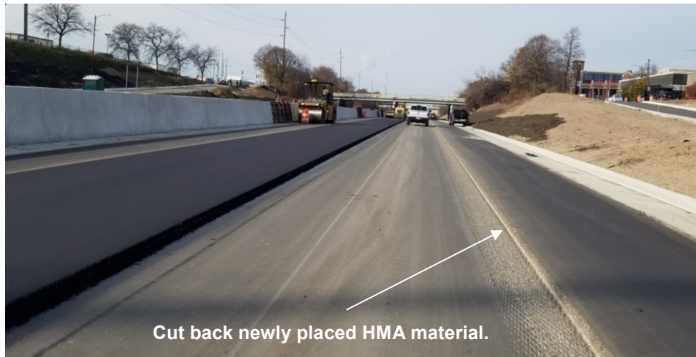
Figure 5.3 Constructing an unconfined joint with cutting back technique at I-496 project, MI
