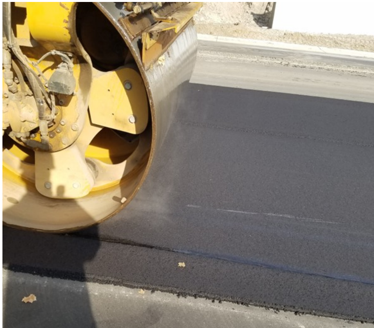
Figure 5.4 Hot pinch rolling method used on the I-496 project, MI, for constructing the confined joint
