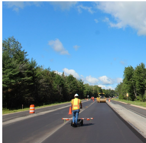
(b) DPS data collection on confined taper joint – Day 2
