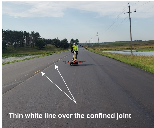
Figure 2.4 Appearance of a thin white line over the confined joint using the Maryland method at the Manning Trail project, MN
