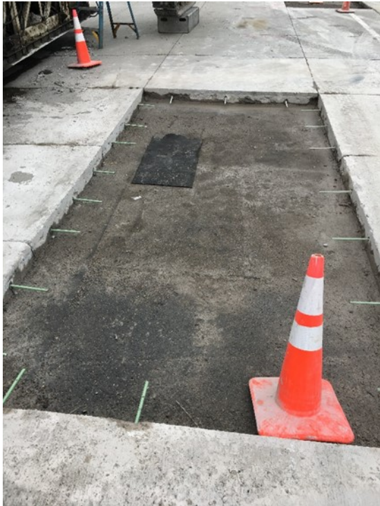
Figure 5.4 shows the placement of concrete in the repaired panels. Concrete was placed with tie bars and bond breaking fabric material.
