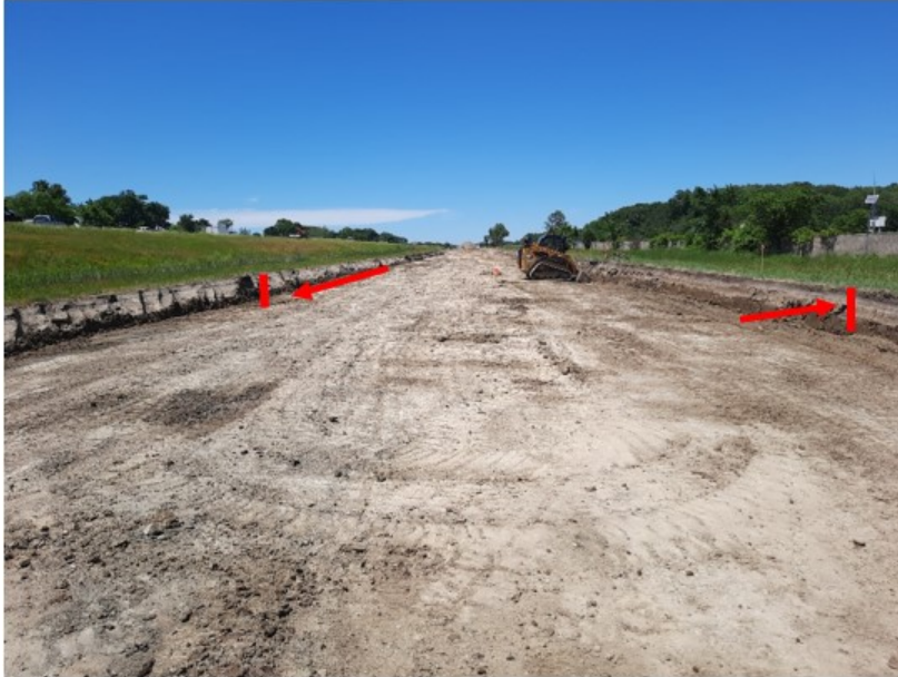
Figure 12-5 Difference in Elevation between the Top Subgrade Layer and the Pavement Edge Level
