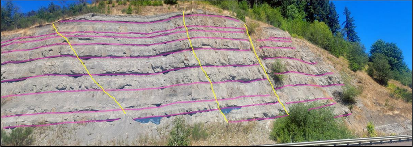
Figure 2.16 Eddyville, Oregon: major discontinuities (yellow) and water seepage areas (blue) in alternating beds of greywacke and siltstone (rose lines mark the bottom of each greywacke bed). Note that this image covers only the extreme east end of the site.
