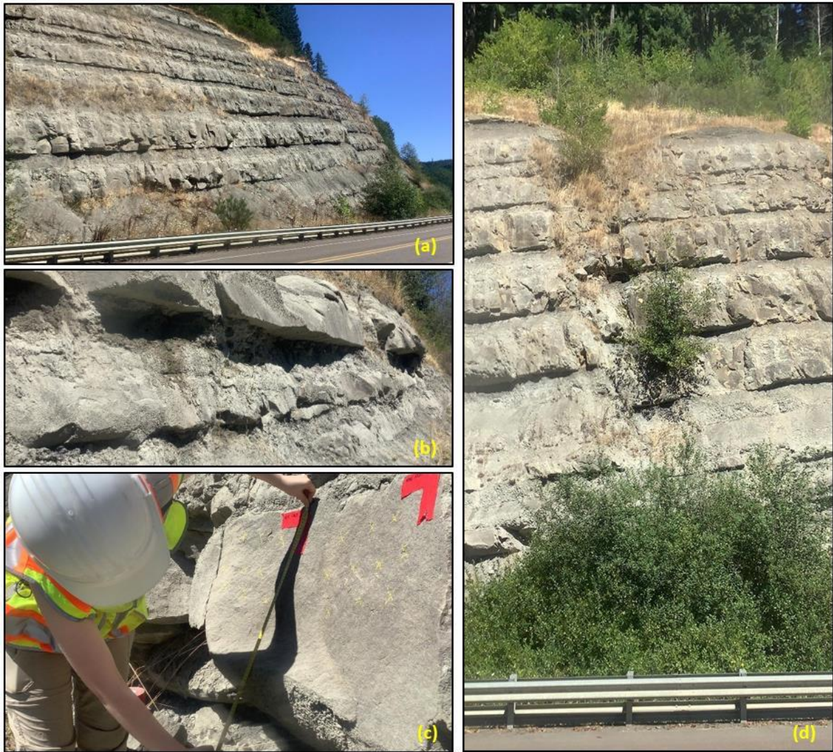
Figure 2.5 Photographs of the geology at the Eddyville research site: (a) view to the east along the highway; (b) example of overhanging greywacke underlain by siltstone with evidence of water seepage; (c) measuring bed thickness at an SH measurement site; (d) high-angle, normal fault with vegetation.
