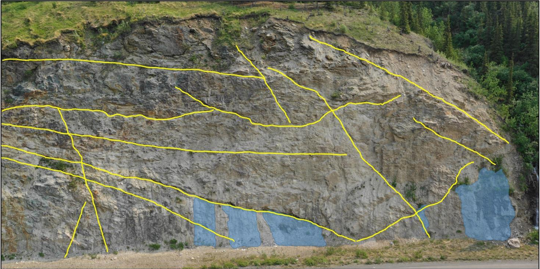
Figure 2.13 Nenana Canyon (MP 241), Alaska, south section: major discontinuities (yellow) and water seepage areas (blue) in micaceous quartzite and muscovite/sericite quartz schist.
