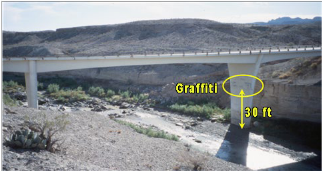
Figure 7.15. Degradation at State Route 147 over Las Vegas Wash, Nevada in 1999.
