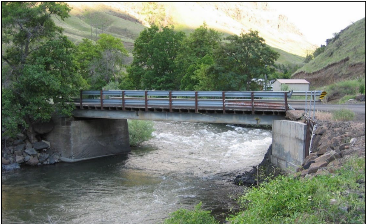
Figure 6.27. View downstream at the Imnaha River Bridge at Lewis Road, Oregon. Image used by permission of WEST Consultants, Inc.
