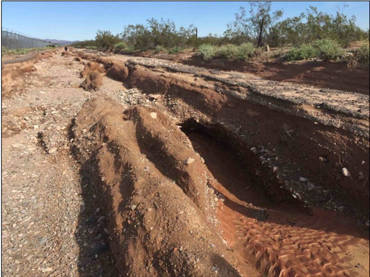
Figure 8.20. Road damage on an alluvial fan caused by locally concentrated overland flow.
