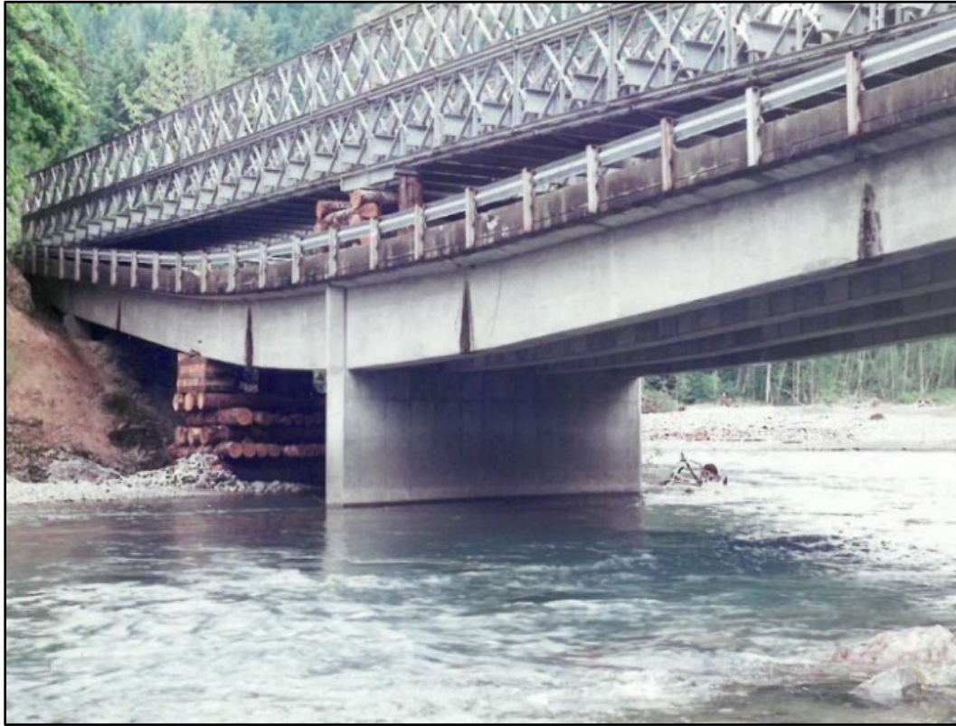
Figure 4.9. Impact of pier scour, leading to structural failure.
