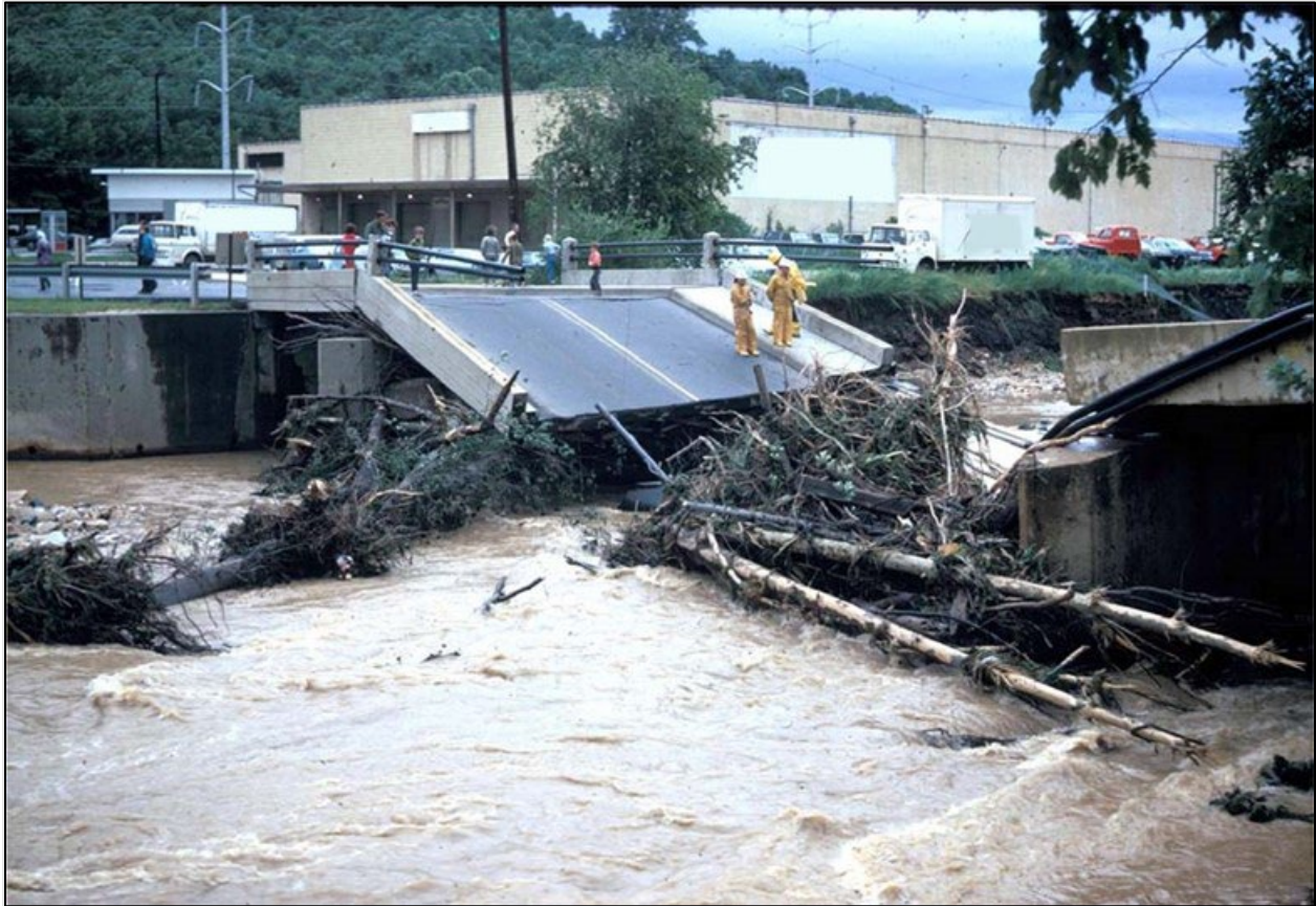
Figure 2.9. Effect of wood accumulation against the closely spaced, in-channel piers of a bridge in New York. Source: FHWA.
