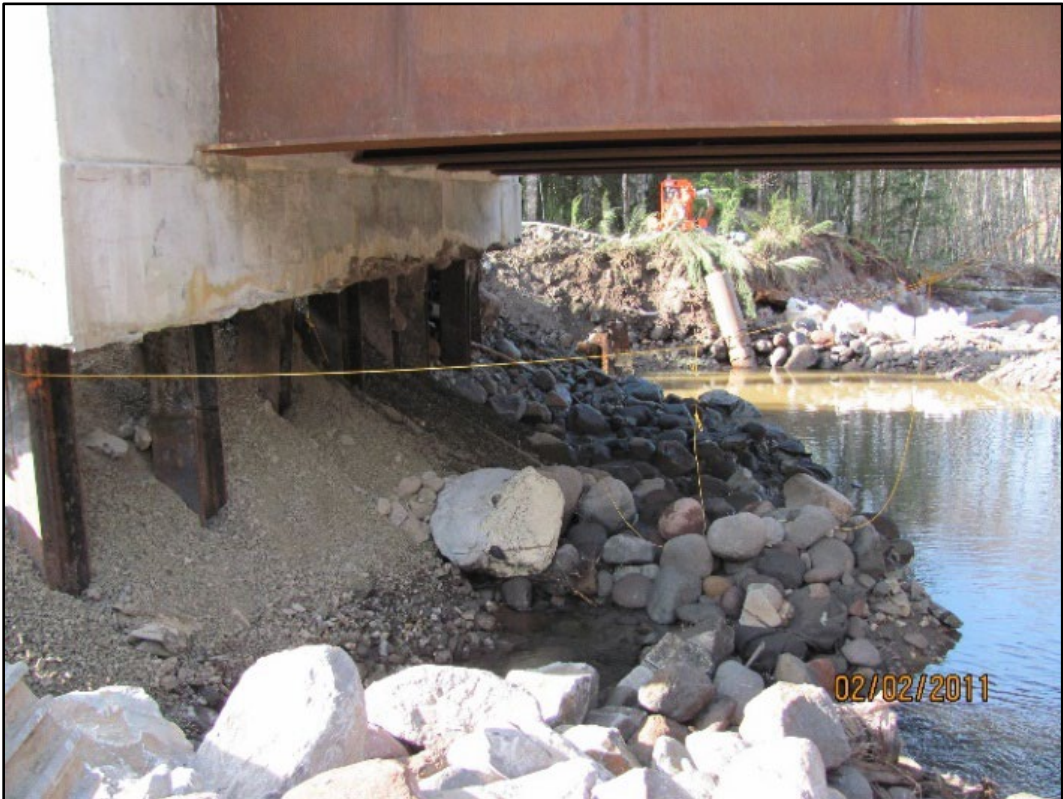
Figure 4.8. Impact of bank erosion on a bridge abutment.
