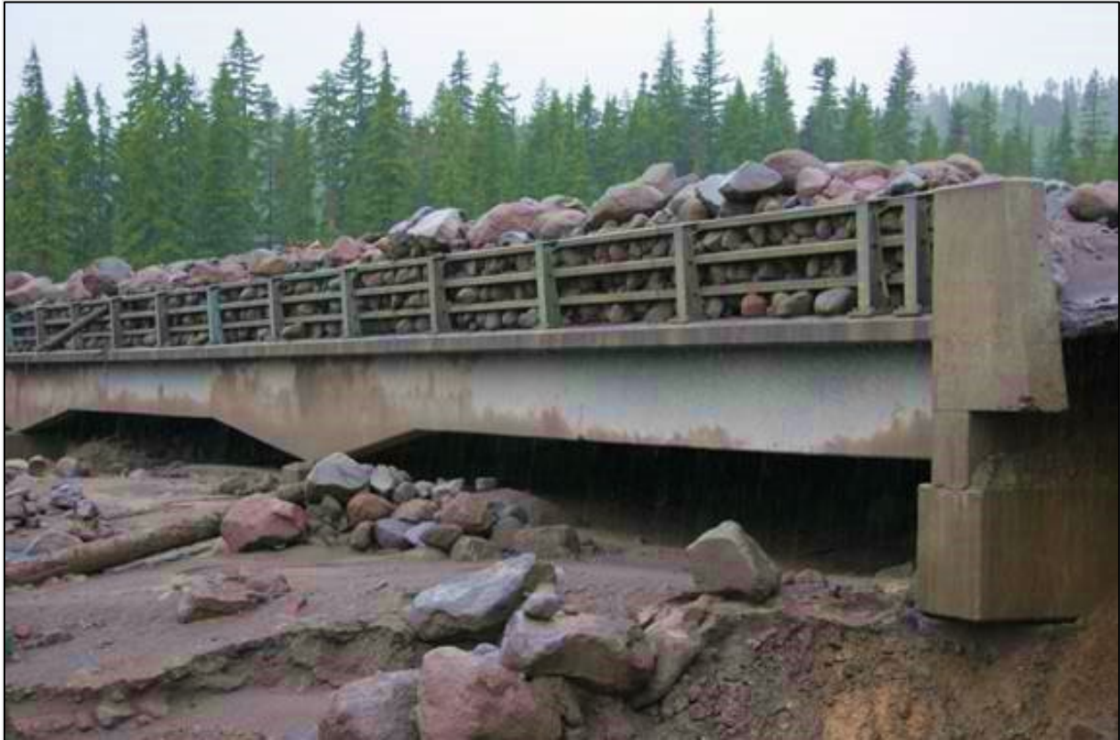
Figure 8.13. Impacts of a combined mud and debris flow on a highway bridge. Source: USFS.
