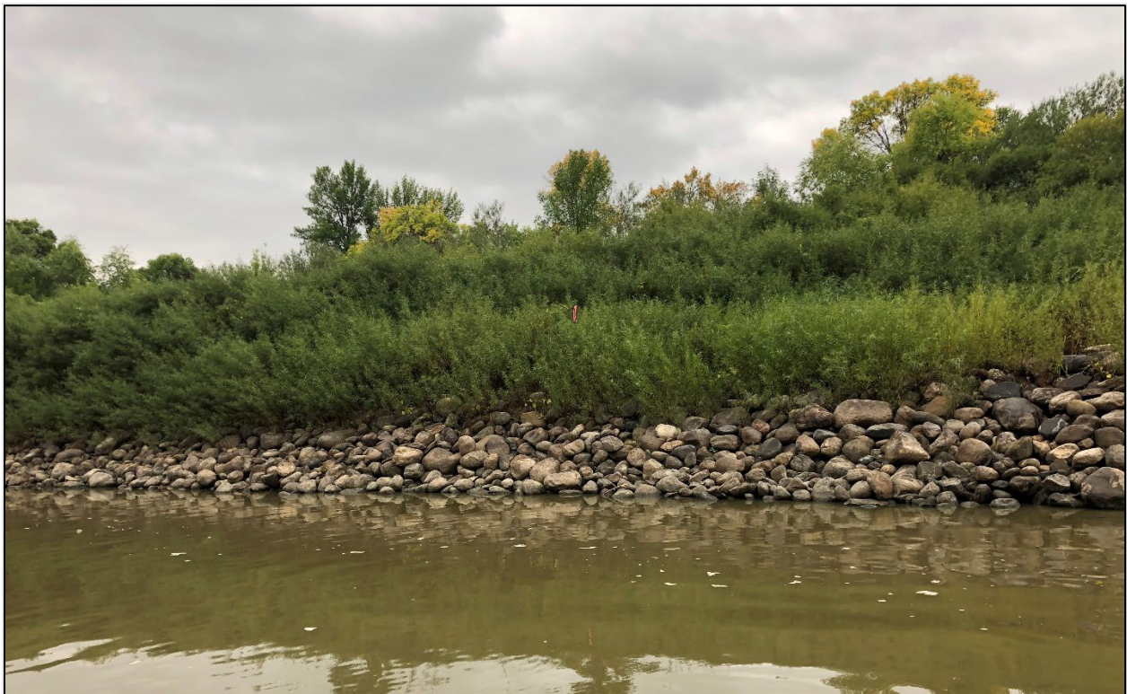
Figure 4.13. Vegetated riprap along the Red River near Fargo, ND. Image used by permission of WEST Consultants, Inc.
