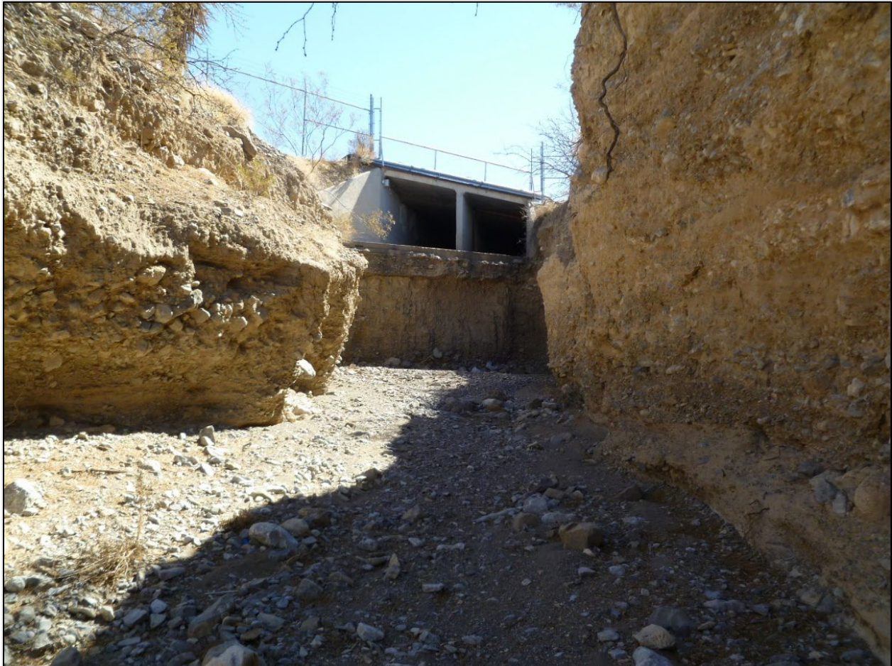
Figure 6.24. Knickpoint at downstream end of a box culvert along Alamogordo Creek, NM. Image used by permission of WEST Consultants, Inc.
