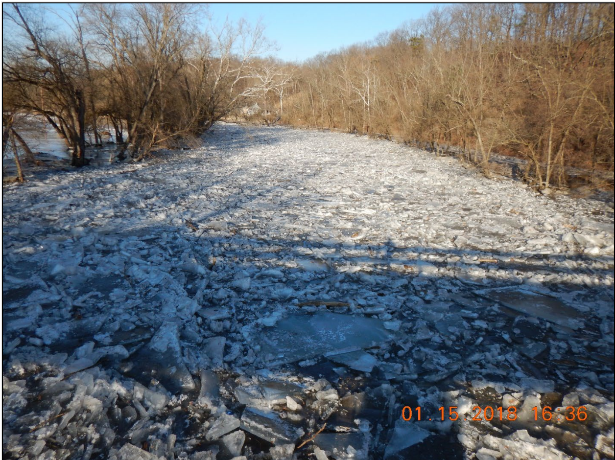
Figure 8.4 Looking upstream along the ice covered Conococheague Creek at a bridge crossing in Williamsport, Pennsylvania. Source: J. Coleman (RK&K) and used by permission.
