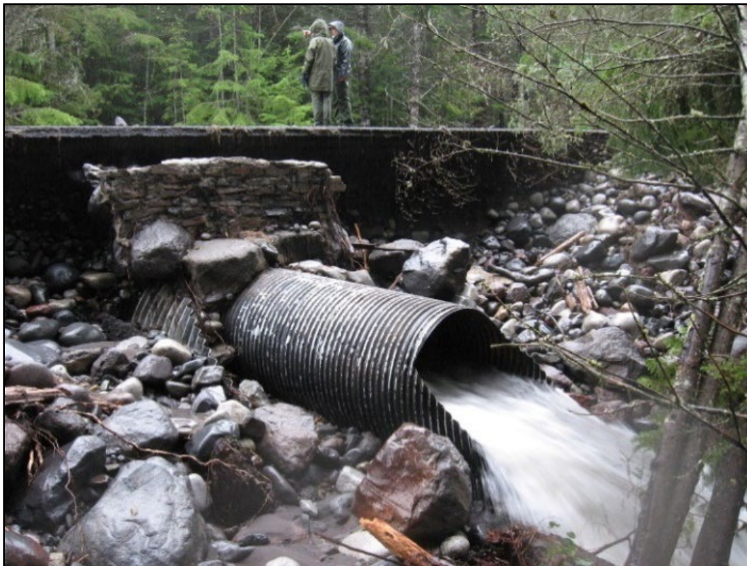
Figure 4.10. Road wash out, a typical impact of culvert overtopping.
