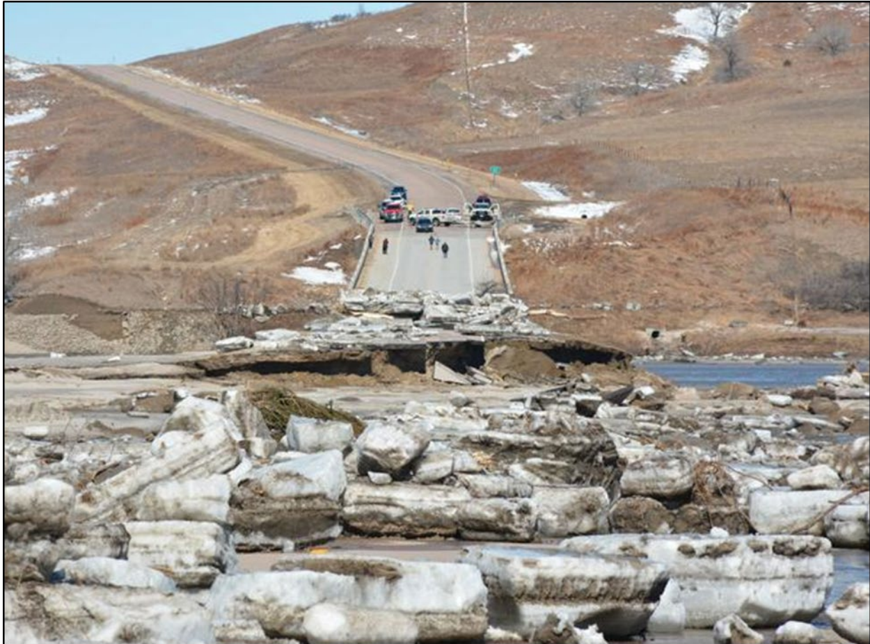
Figure 8.5. In 2019, ice floes destroyed the Highway 281 bridge over the Niobrara River in Nebraska. Image used by permission of T. Miles (© 2019).
