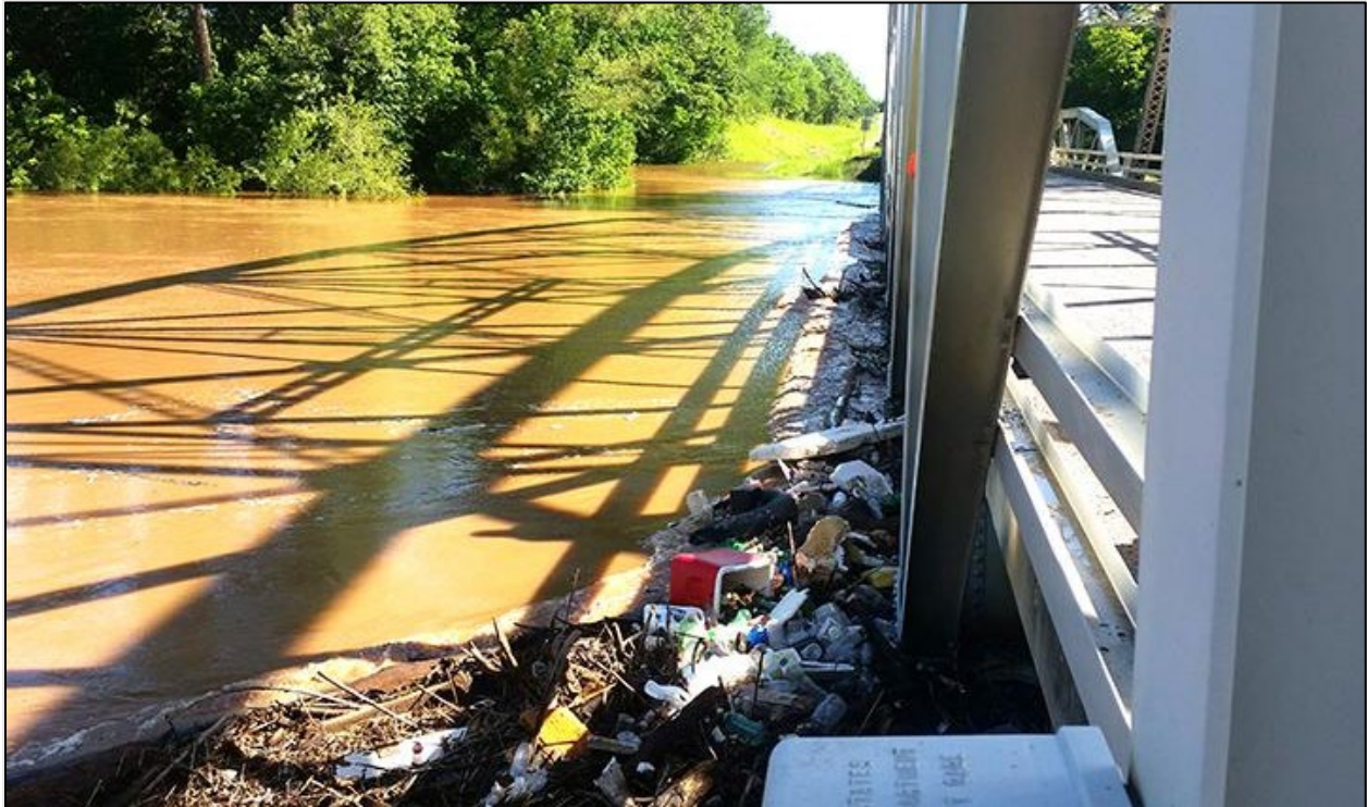
Figure 8.9. Litter and trash accumulation (SH-99 Washita River Bridge, Oklahoma). Image used by permission of the Oklahoma Department of Transportation.
