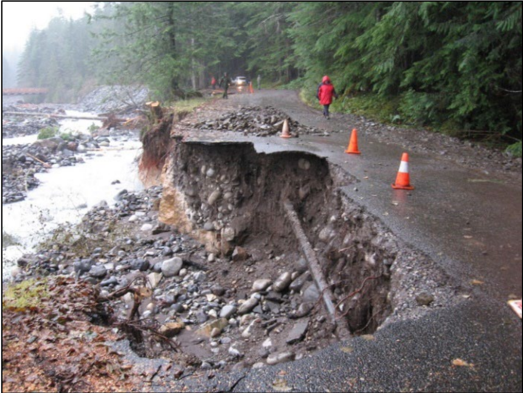
Figure 4.7. Impact of bank erosion on a road running along the river corridor.
