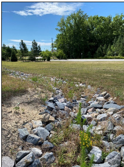
Figure 1. Example of rip-rap lining eroding channel downslope of pipe outlet
