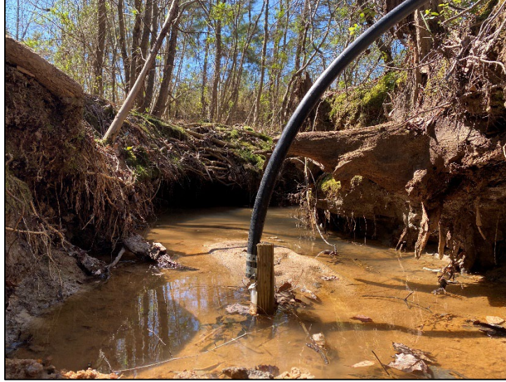
Figure 25. Evidence of unstable undercuts at MP467
