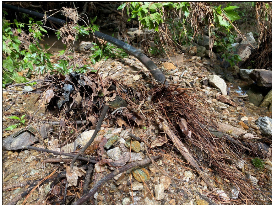
Figure 18. MP459 equipment buried by sediment transported during 2.99 in storm
