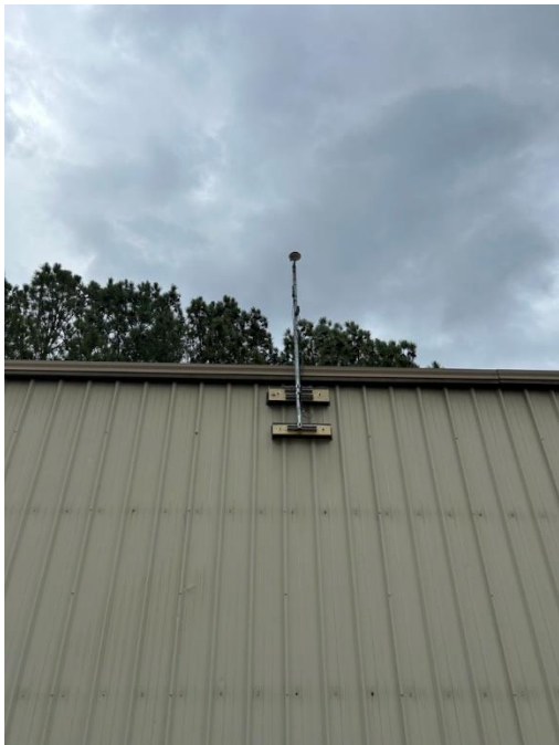
Figure 4. GNSS antenna installed on the roof of the shuttle's storage and charging location in Cary's Bond Park. (Image courtesy of Beep)
