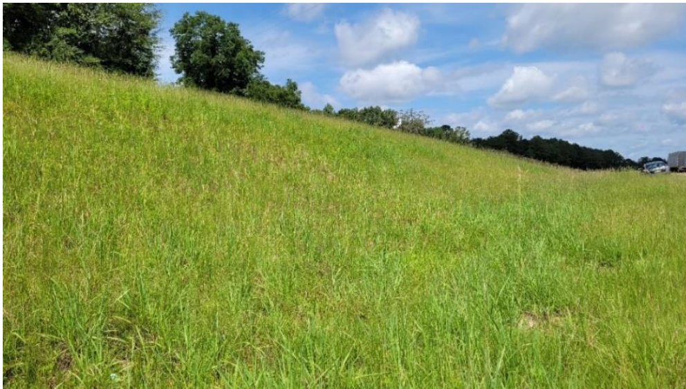
Figure 2.7 Vetiver stabilizing a previously failed highway slope in Mississippi.
