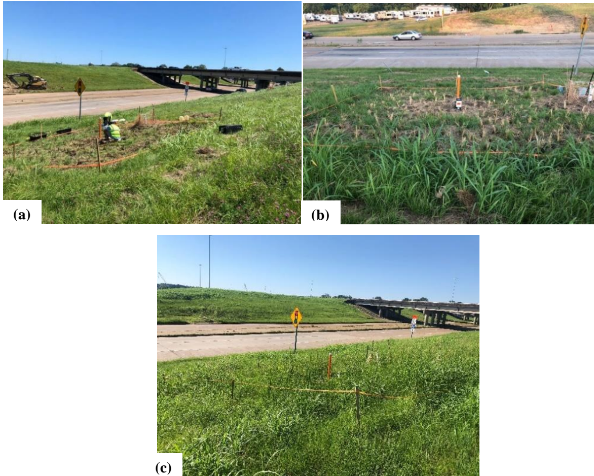
Figure 4.12 Planting vetiver on highway embankment at Terry Rd: (a) looking southwest from reinforced section, (b) looking southwest at reinforced section after vetiver has achieved a few weeks' growth, and (c) looking southwest from reinforced section in October 2020
