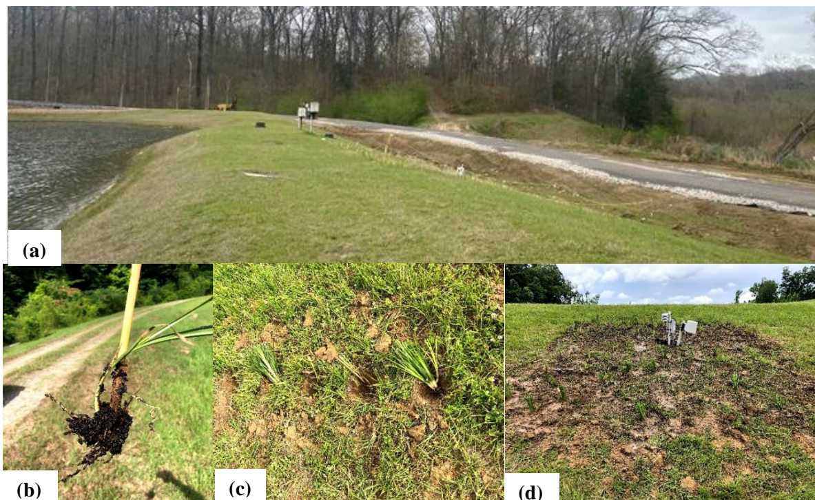
Figure 4.2 Planting vetiver on test levee at ERDC: (a) looking east, (b) vetiver tiller before planting, (c) planted vetiver, and (d) looking north after planting
