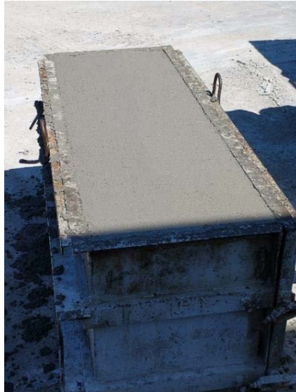
Figure 2.27: Placement of Second Truckload in Second Trial Placement (Containing Set Retarding Admixture) with No Observable Air Pockets on the Concrete Surface
