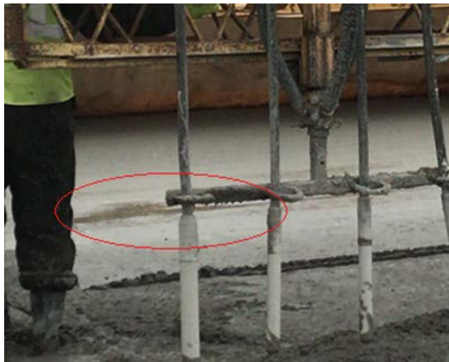
Figure 2.44: Ponded Water on the Surface of the Bridge Deck
