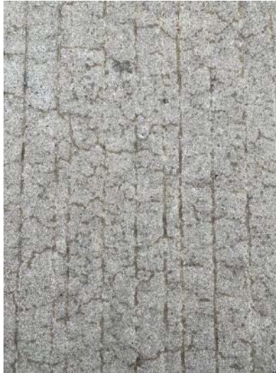
Figure 3.26: Map Cracking on a Typical Section of MN-IC-LC-HPC-9
