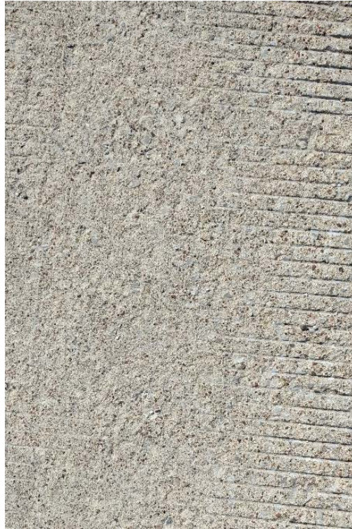
Figure 3.33: Scaling Damage Observed Near the Shoulders of KS-IC-LC-HPC-1 (Survey 3)
