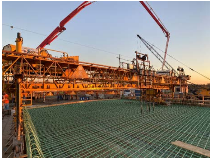
Figure 2.50: Consolidation and Finishing Equipment
