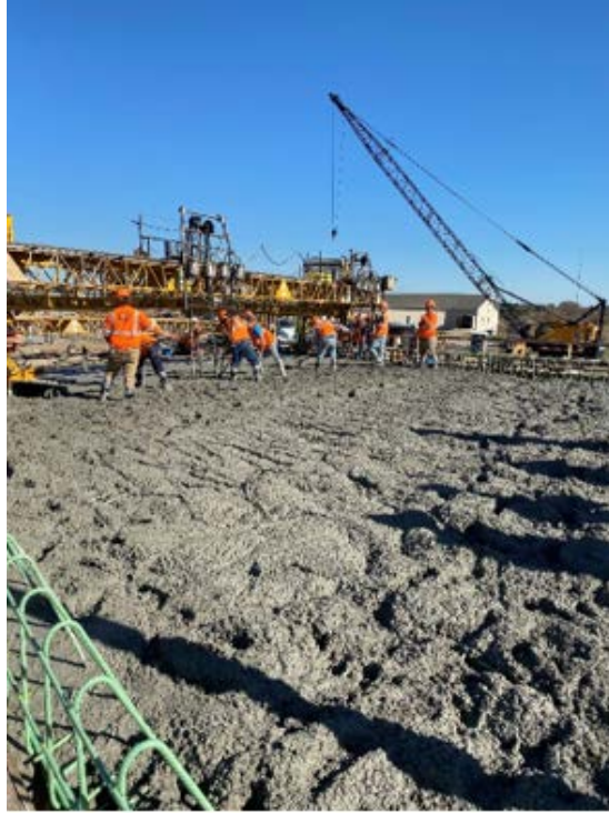
Figure 2.52: Concrete Left Unconsolidated and Unprotected Due to Inoperable Roller Screenshot
