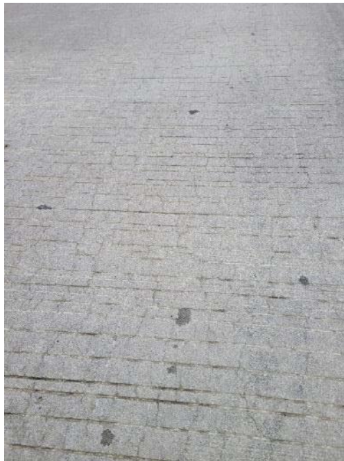
Figure 3.23: Map Cracking on a Typical Section of MN-IC-LC-HPC-8
