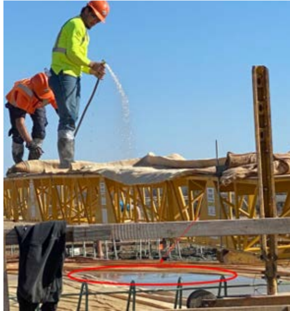
Figure 2.55: Ponding Observed on the Deck
