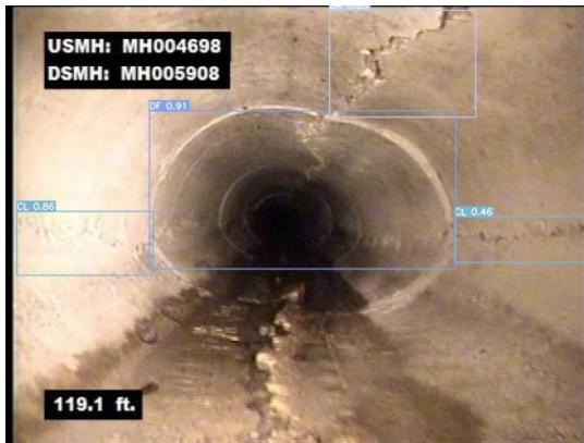
(a) Longitudinal cracks and deformation
