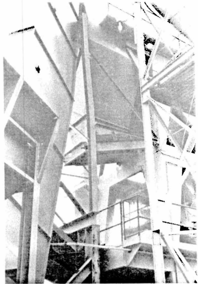
FIGURE 6 Surge Hopper and Drag-Out Belt
