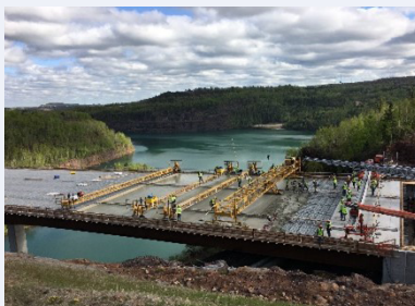
Bridge deck pour on the TH 53 relocation project over the Rouchleau Pit in Virginia, MN
