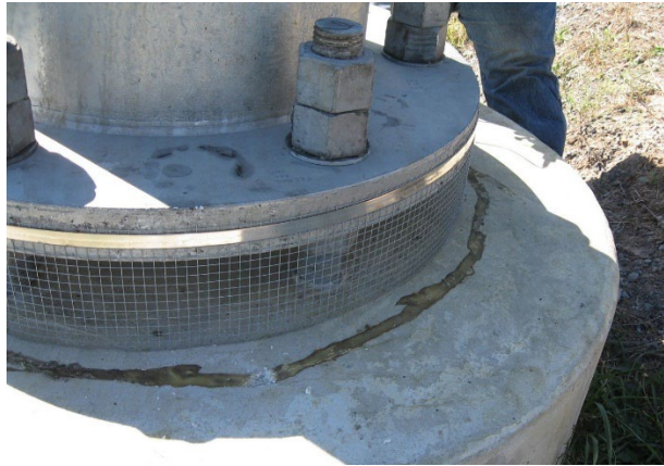
Figure 88. Photo. Gravity filled crack on the top face of a foundation.
