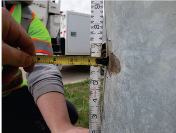
Figure 73. Photo. Impact damage to end support.
