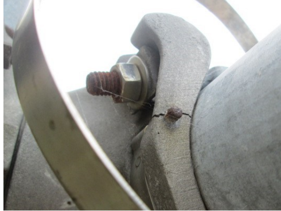
Figure 78. Photo. Crack to cast aluminum clamp supporting a traffic signal.
