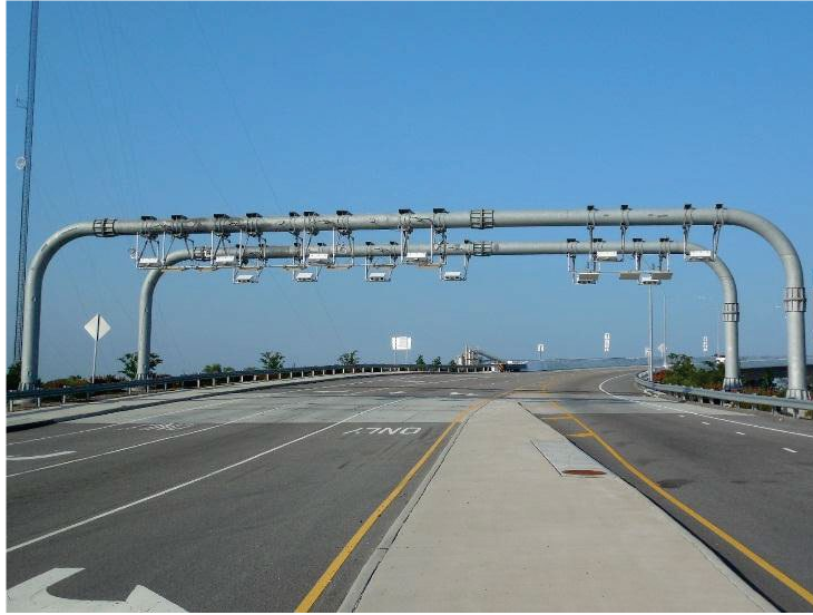
Figure 7. Photo. Two monotube overhead span structures.
