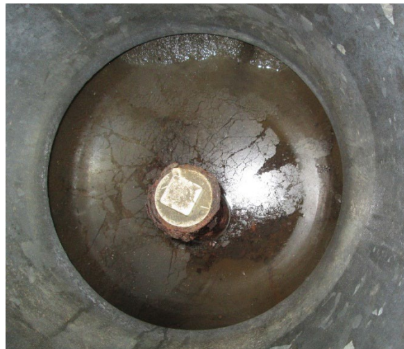
Figure 89. Photo. Standing water accumulated inside a vertical support.
