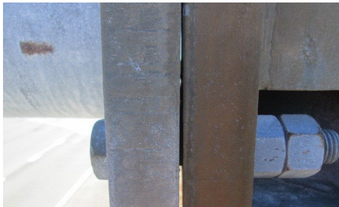
Figure 104. Photo. Gap between faying surfaces.
