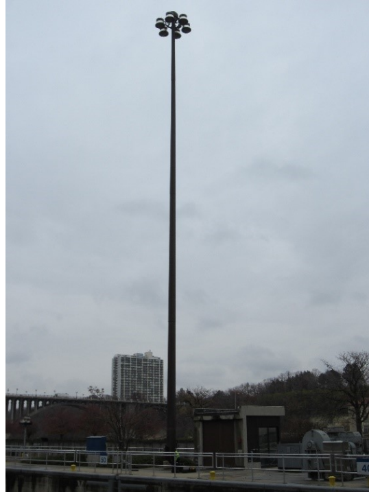
Figure 19. Photo. High mast light structure.
