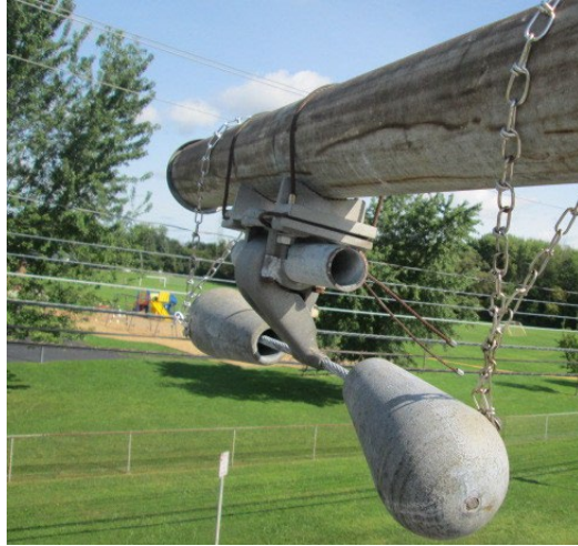
Figure 107. Photo. Damper at mast arm end span. Chains restrict full motion.
