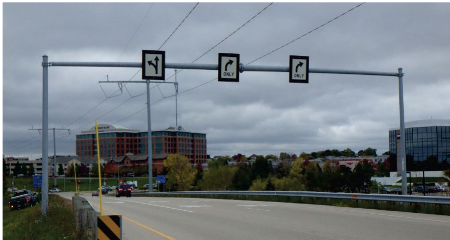
Figure 6. Photo. Overhead span, single chord and pole structure.
