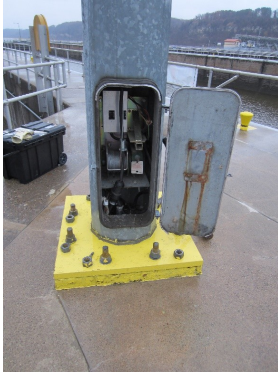
Figure 20. Photo. High mast light winch system.
