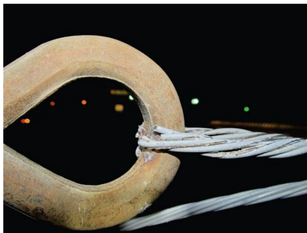
Figure 79. Photo. Broken wires at span wire connection to post.
