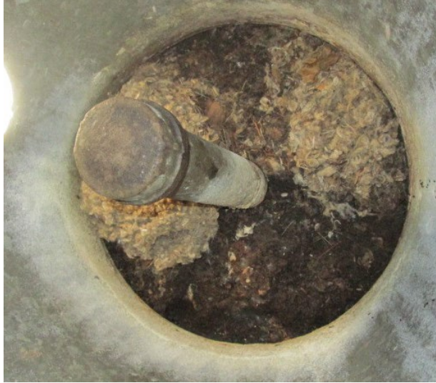
Figure 91. Photo. Rodent nesting debris inside the base of a vertical end support.
