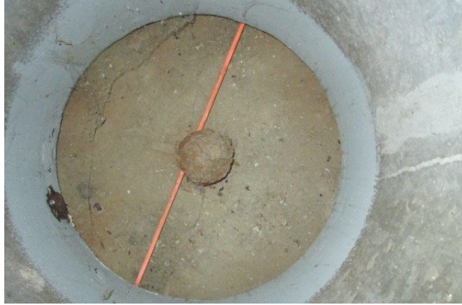
Figure 97. Photo. Interior of a vertical end support showing painted repair and inspector's probe rod.
