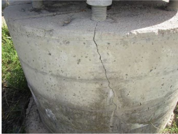
Figure 68. Photo. Foundation cracks protruding into foundation from anchor rod.
