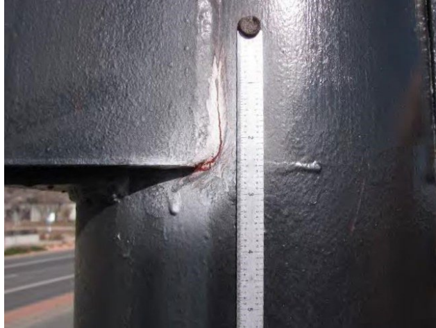
Figure 74. Photo. Cracked weld at end support connection weld.
