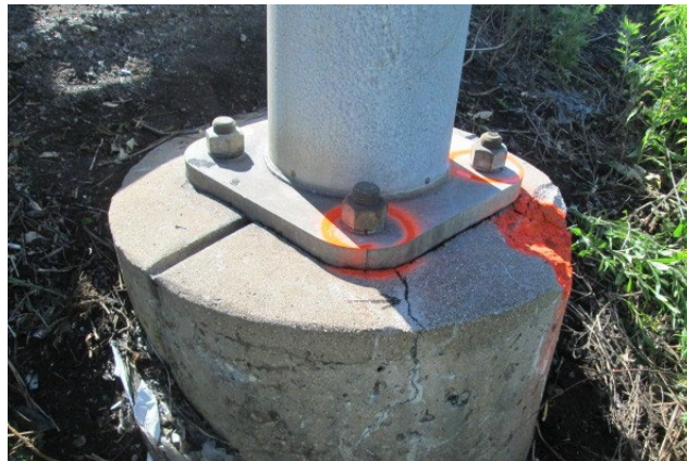
Figure 87. Photo. Deteriorated foundation showing crack and edge spalling.
