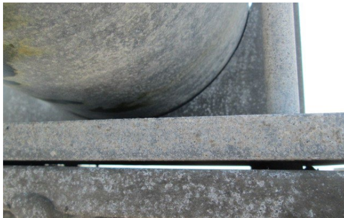
Figure 101. Photo. Gap between horizontal saddle and support beam.
