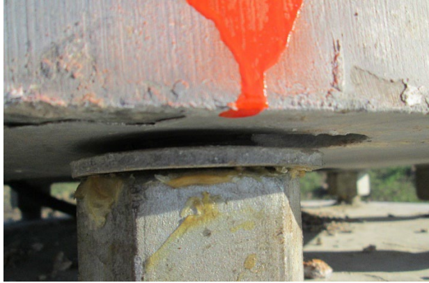
Figure 92. Photo. Gap between leveling nut and base plate.
