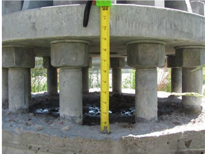
Figure 70. Photo. Anchor rod unsupported length above tolerance.
