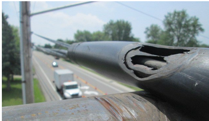
Figure 54. Photo. Exposed wires due to wear.
