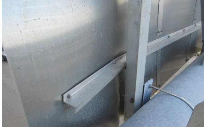
Figure 111. Photo. Impact damage to flat panel and wind beam.
