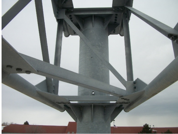
Figure 42. Photo. Cantilever truss connection with horizontal plates on post support and chords.
