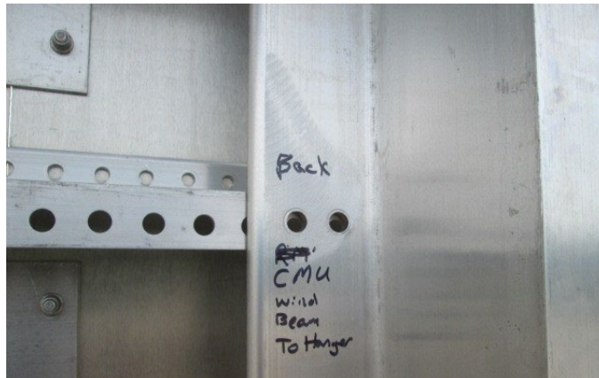
Figure 108. Photo. Missing wind beam to hanger connection bolts.
