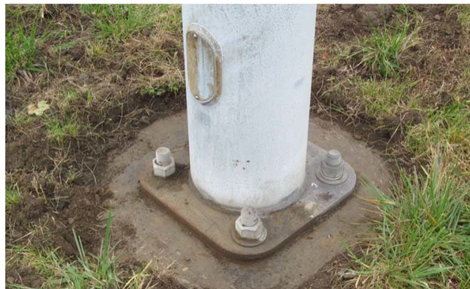
Figure 31. Photo. Base plate mounted directly onto concrete without leveling nuts.
