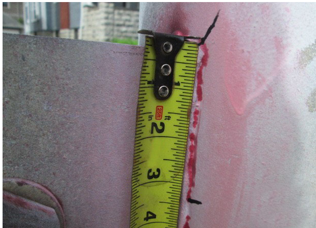
Figure 85. Photo. Dye penetrant used to highlight cracked connection.
