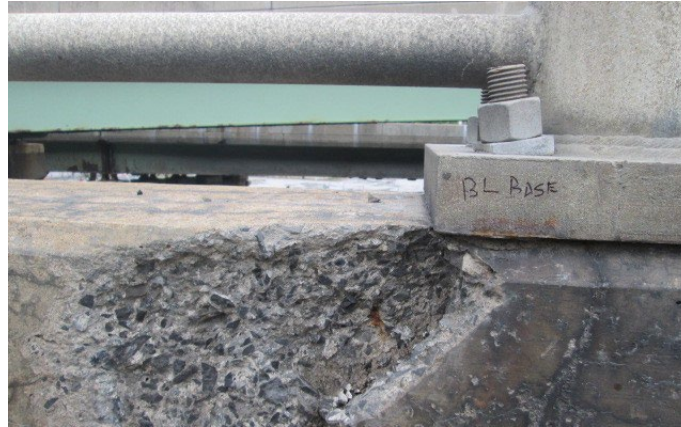
Figure 93. Photo. Out-of-plumb anchor rod repaired with a beveled plate washer.
