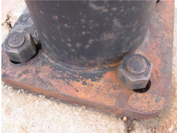
Figure 71. Photo. Oversized holes in base plate.
