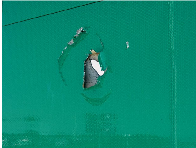
Figure 77. Photo. Damage to reflective coating of overhead sign panel.
