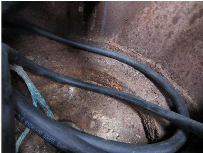
Figure 72. Photo. Corrosion to uncoated weathering steel post interior.
