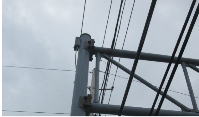
Figure 55. Photo. Overhead lines near structure to be inspected.
