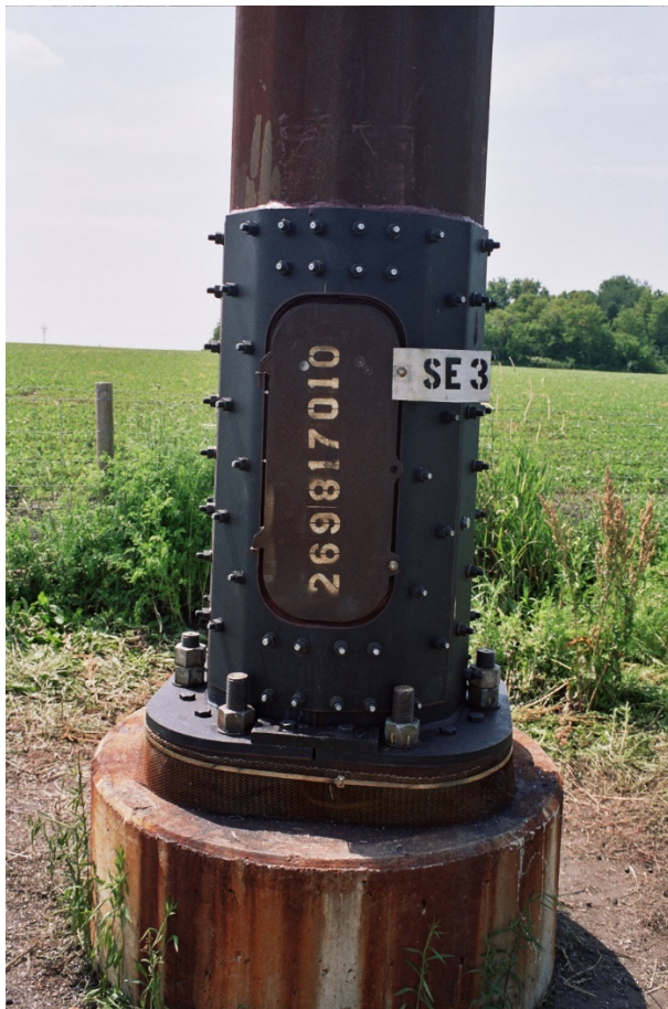
Figure 100. Photo. Clamshell repair at the base of a high mast light pole.
