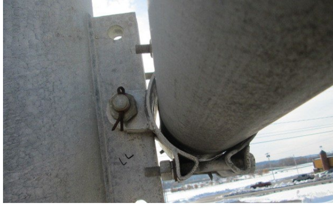
Figure 103. Photo. Gap between chord and clamp assembly.
