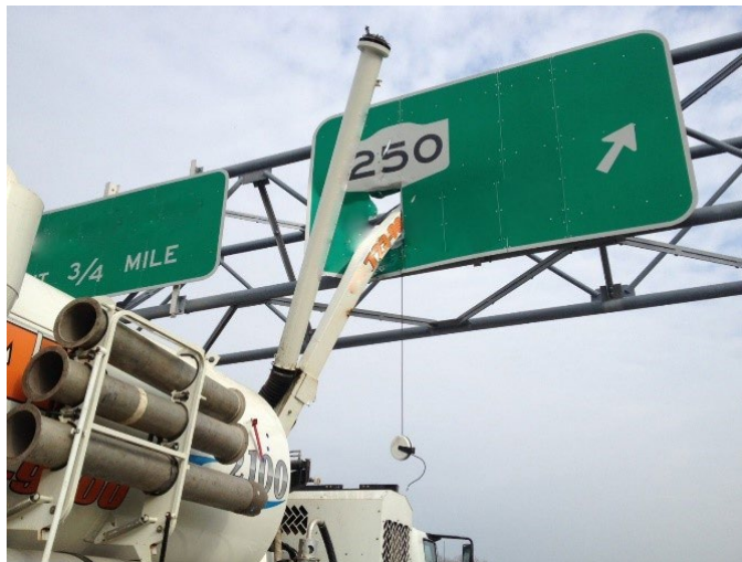
Figure 112. Photo. Impact damage to sign panel.
