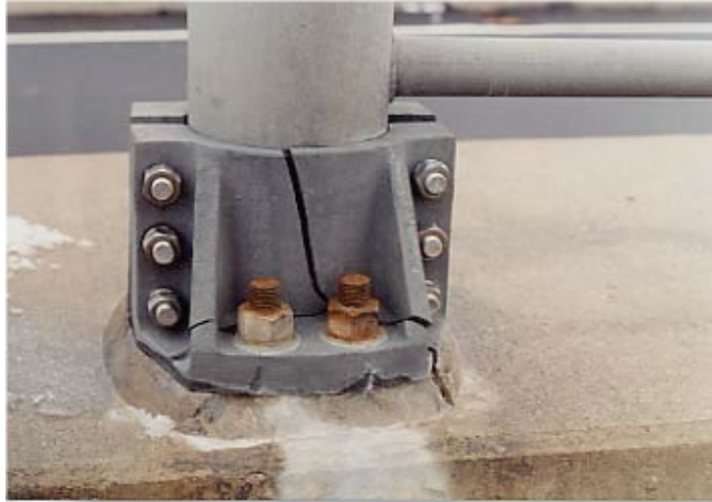
Figure 32. Photo. Cracked aluminum casting clamp.
