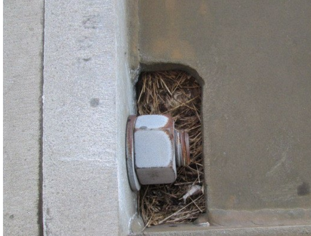
Figure 105. Photo. Nesting debris accumulation inside the connection assembly.
