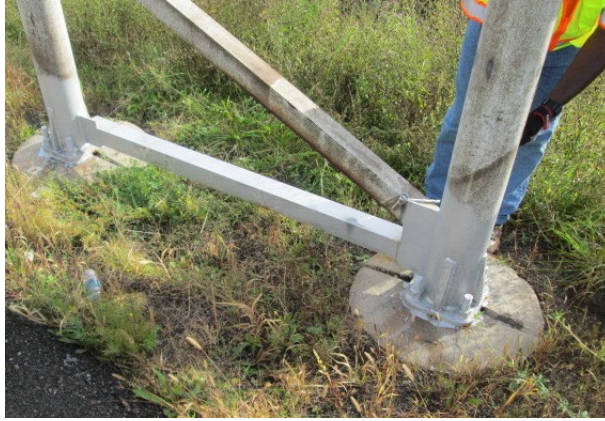
Figure 99. Photo. Stiffener addition repair at the base of a vertical end support frame.
