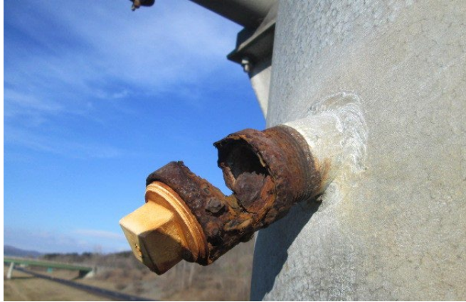
Figure 96. Photo. Damaged conduit nipple with aftermarket polyvinyl chloride plug.
