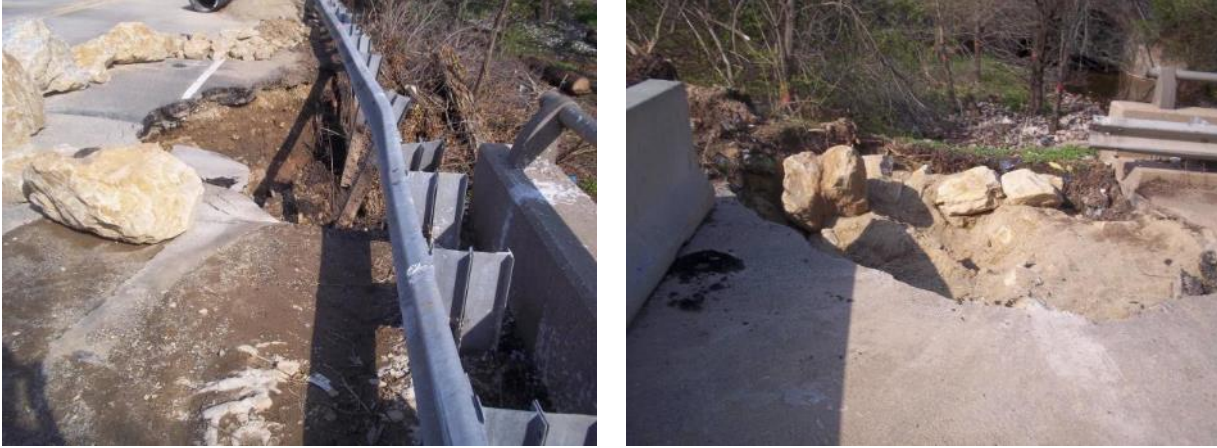
Figure 2.10. Sinkhole damage to the Plymouth Road Bridge near Plymouth Township (August 2015).
