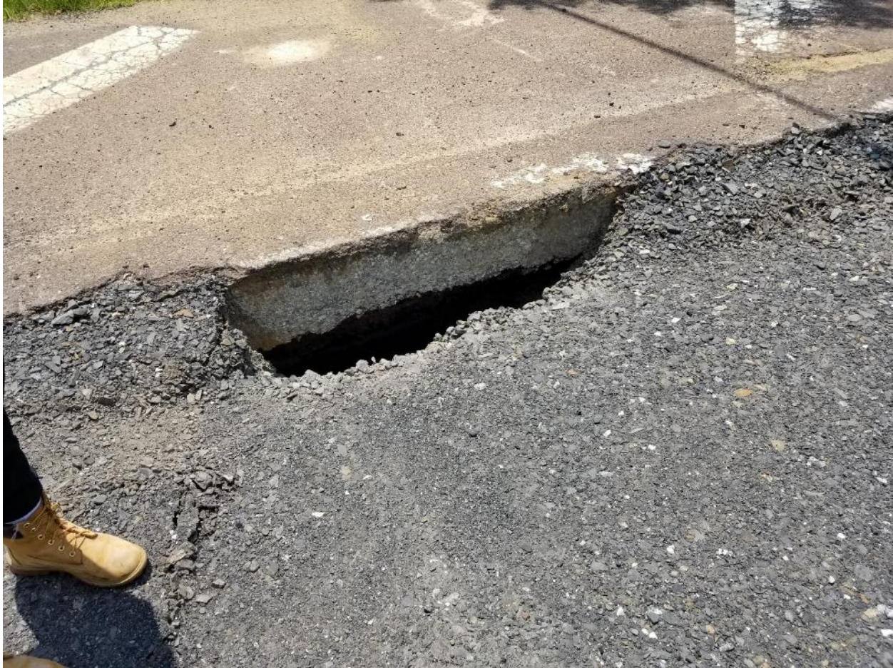
Figure 5.4. Evidence of void features at Sinkhole 2.
