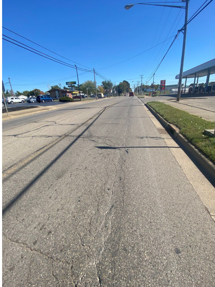
Figure 3.3 Typical Distresses on PIC-22-18.42
