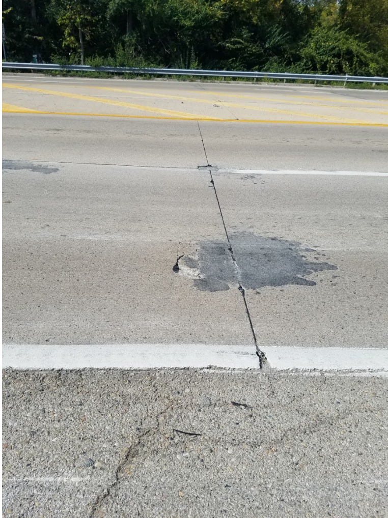
Figure 3.8 Joint Spalling, GRE-44-7.91
