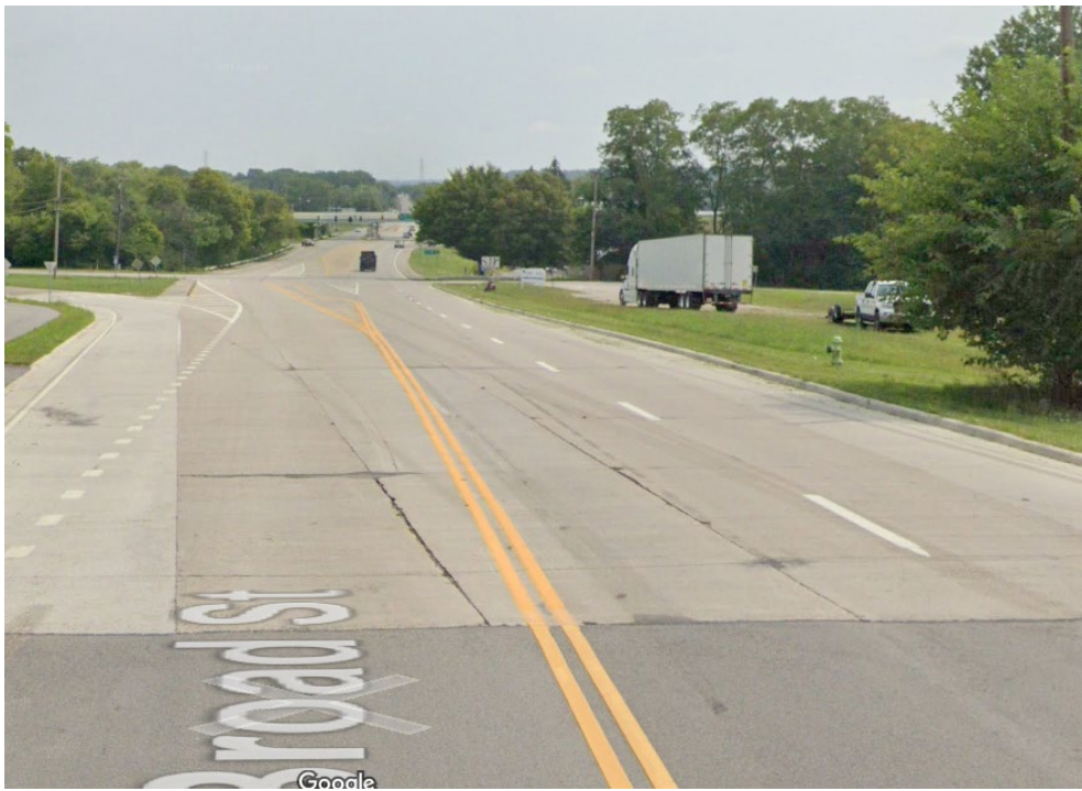
Figure 3.10 Longitudinal Joints within the travelled lanes (Google Maps, 2021)
