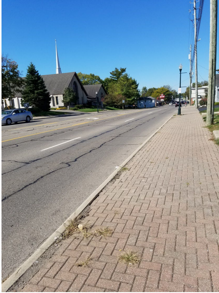
Figure 3.2 Typical Distresses on FRA-317-18.54
