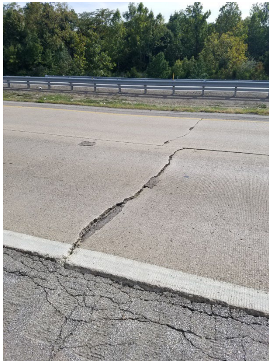
Figure 3.4 Typical Failed Transverse Crack on GRE-35-0.00
