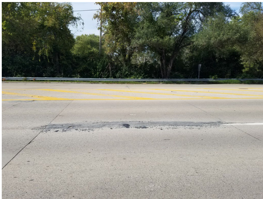
Figure 3.7 Patched Longitudinal Spalling, GRE-444-7.91
