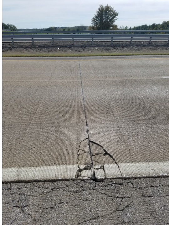
Figure 3.5 Failing Joint on GRE-35-0.00
