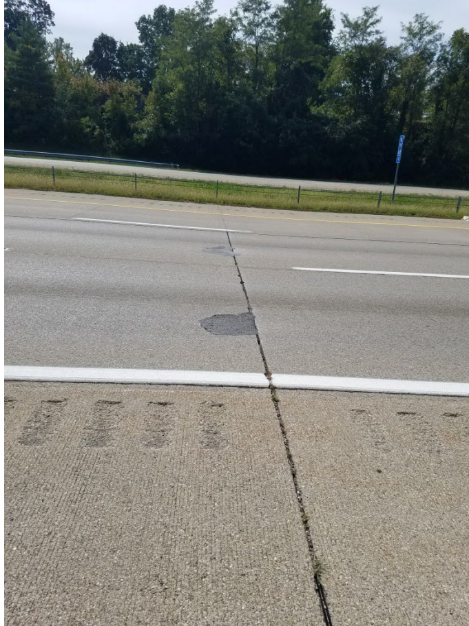
Figure 3.7 Joint Spalling and Repairs on HAM-275-36.58
