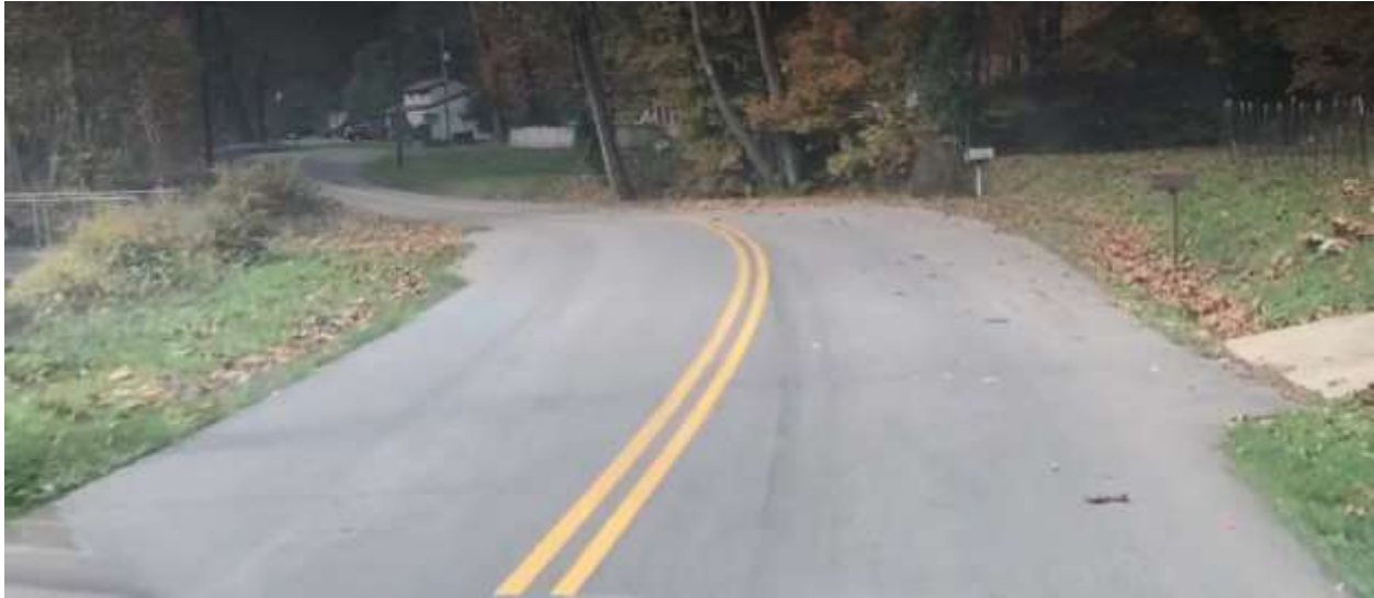
Figure D.9 Pictures taken during evaluation of Bonser Run Road
