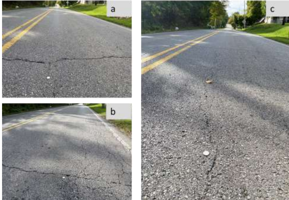
Figure D.4 Pictures taken during evaluation of Licking County section 2 (a) Transverse cracks, (b) Longitudinal cracks (c) Alligator crack
