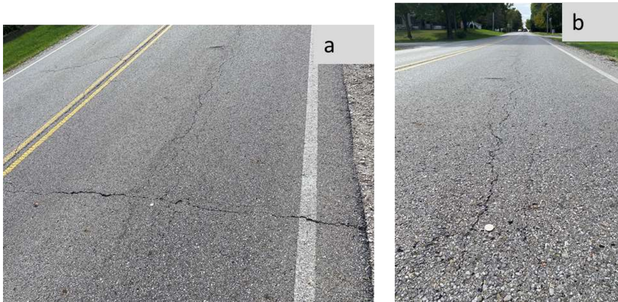
Figure D.3 Pictures taken during evaluation of Licking County section 1 (a) Transverse cracks, (b) Longitudinal cracks
