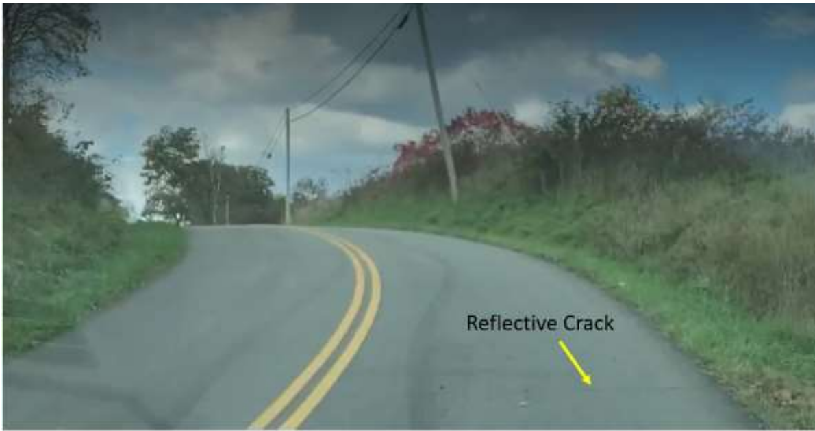
Figure D.13 Pictures taken during evaluation of Bussey Road in Scioto County
