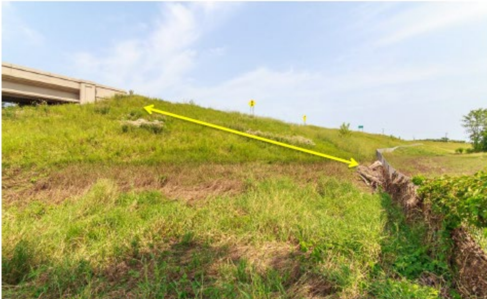
Fencing on the right of way line should of been turned up at the abutment. With the standard practice of running the ROW fence to the waterline, there is no encouragement to go under the bridge (note the fence also caught flood debris).
