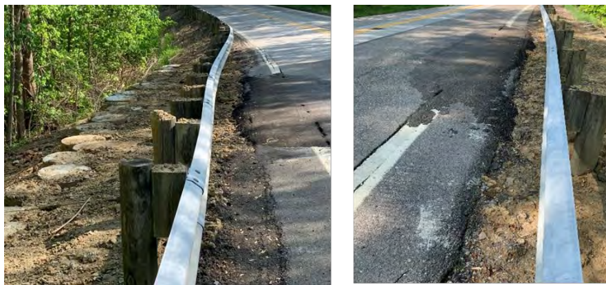
(b) Bending in guardrail.
