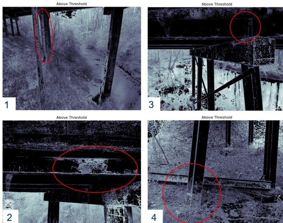
Figure 13. Photographs. Results of entropy thresholding. Circles = corrosion.
