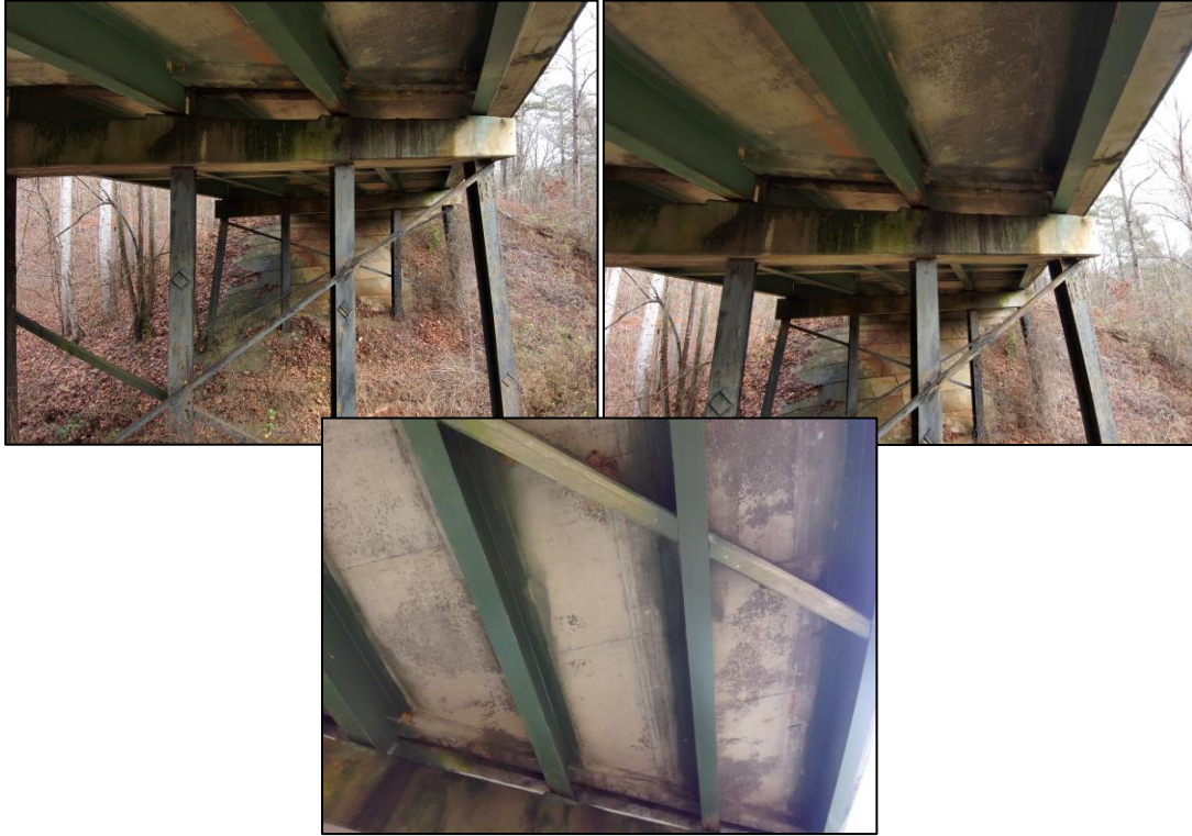
Figure 4. Photographs. Underside of the Bear Creek bridge deck at (a) 0° rotation (b) 50° rotation and (c) 80° rotation.
