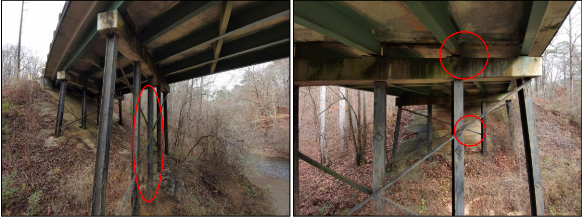
Figure 3. Photographs. Bridge over Bear Creek, Douglasville. Red circles = identified corrosion.
