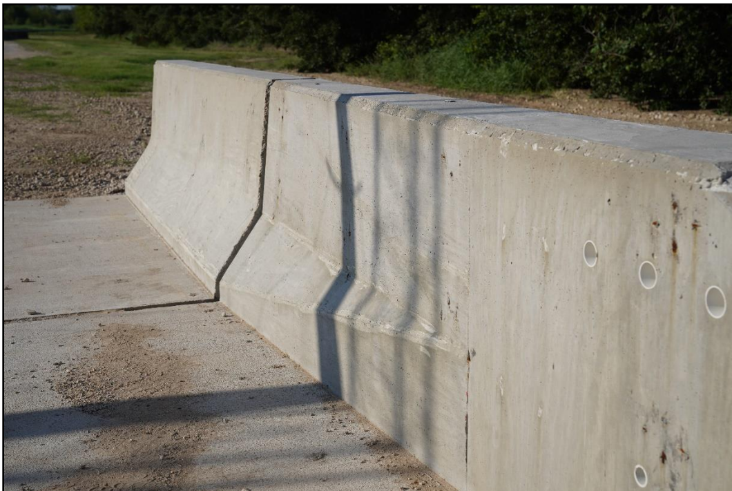
Figure 6.3. Concrete Parapet Shape Transition at Impact Prior to Testing 611801-03-1&2.
