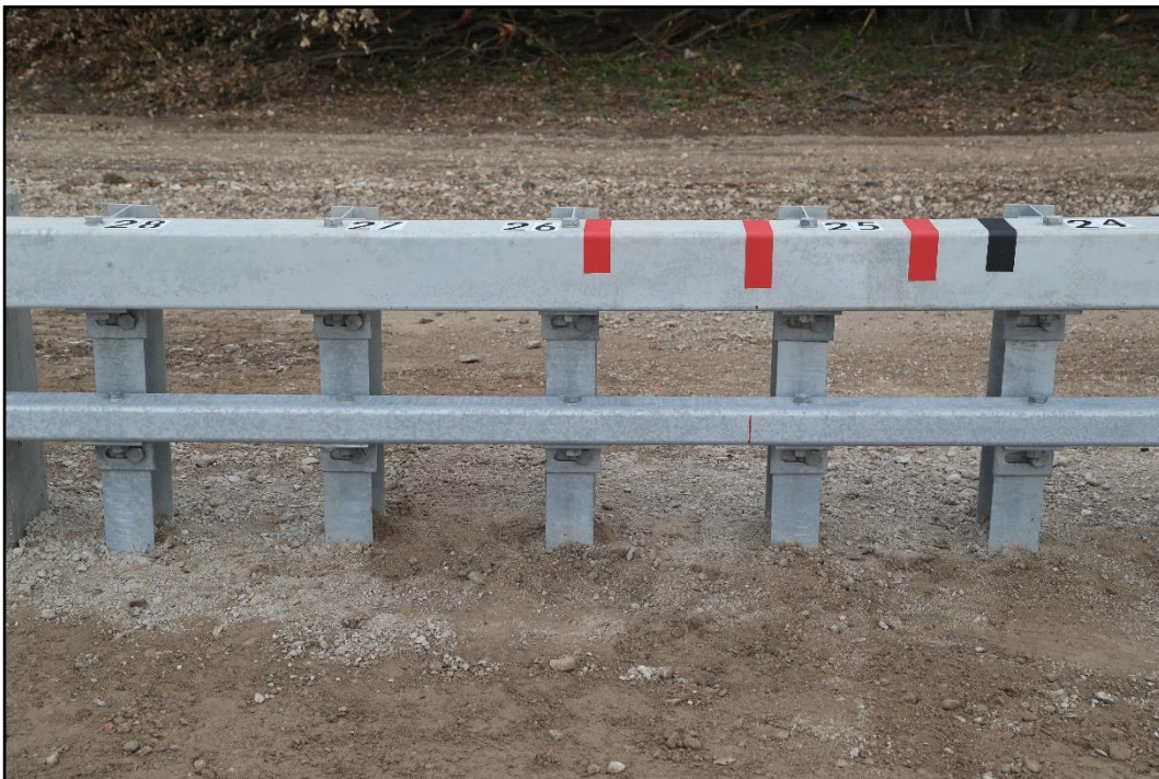
Figure 7.3. Box Beam Guardrail Transition to Concrete Parapet at Impact Prior to Testing 611801-04-1&2.
