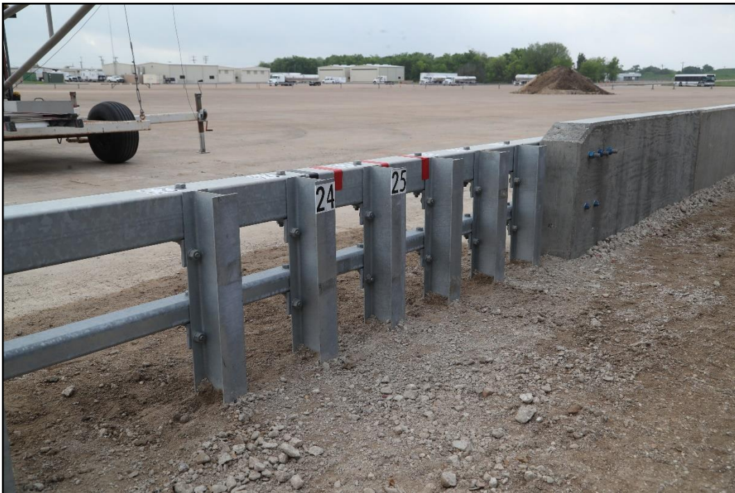
Figure 7.5. Field Side of the Box Beam Guardrail Transition to Concrete Parapet prior to Testing 611801-04-1&2.
