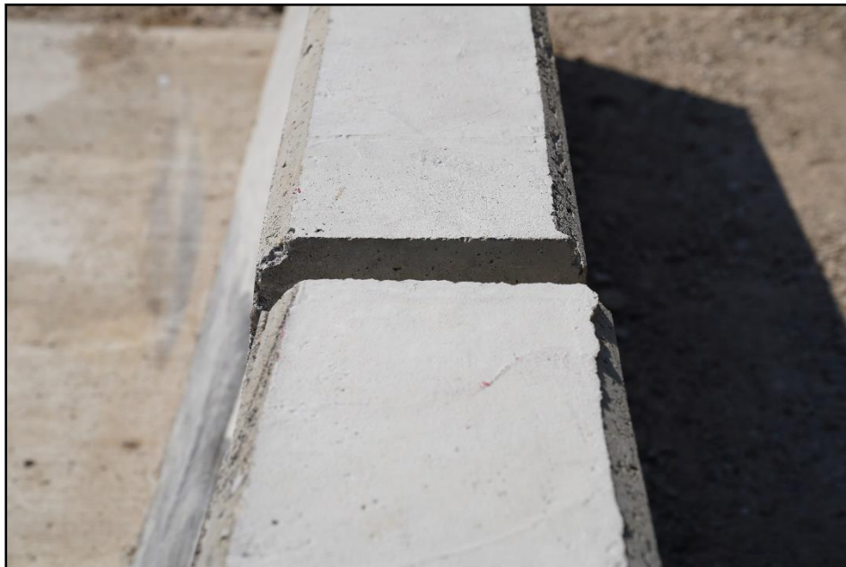
Figure 6.11. Concrete Parapet Shape Transition after Test at the Parapet Joint 611801-03-1.
