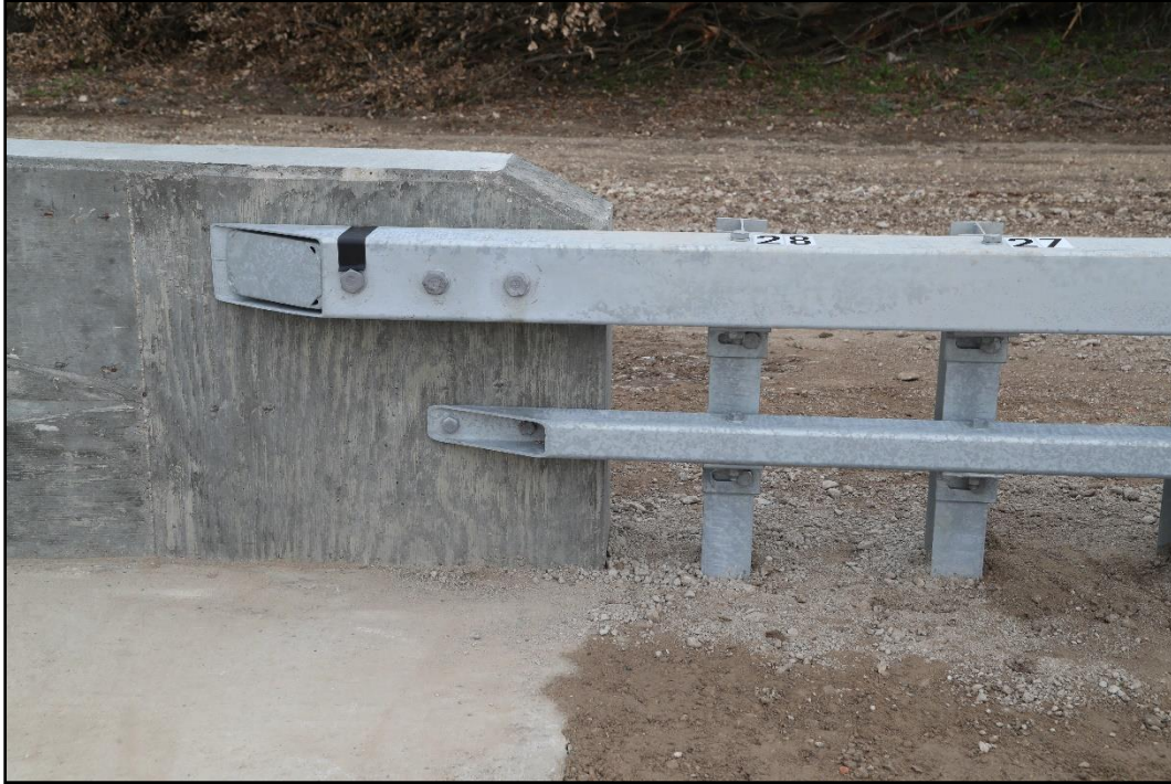
Figure 7.4. Box Beam Guardrail Transition to Concrete Parapet at the Box Beam Transition prior to Testing 611801-04-1&2.
