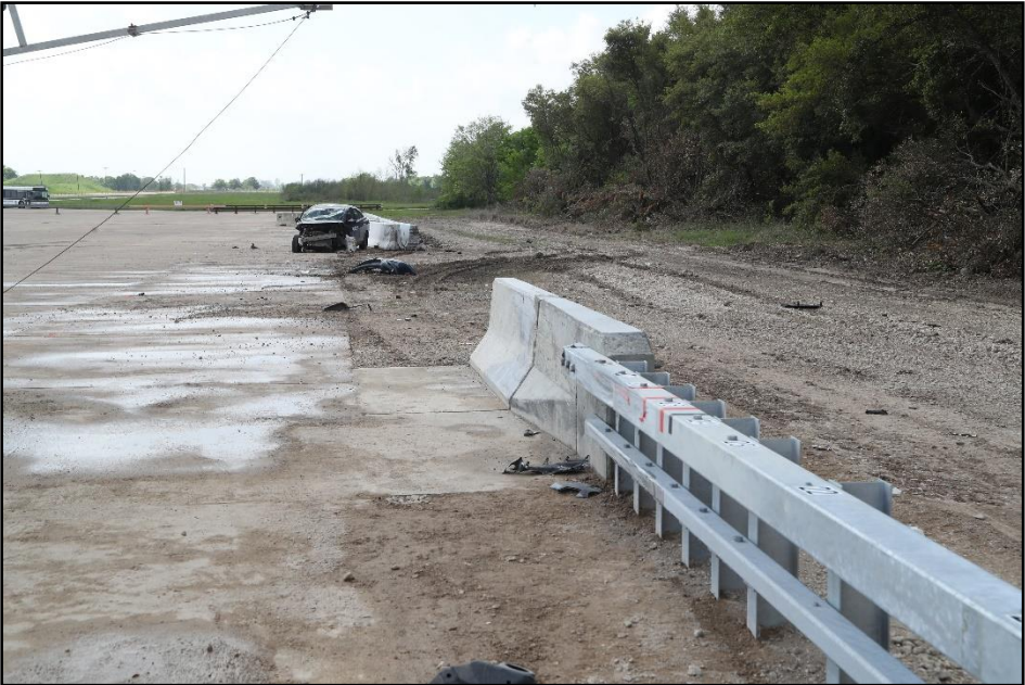
Figure 7.11. Overall View of the Box Beam to Concrete Barrier Transition after Test 611801-04-1.
