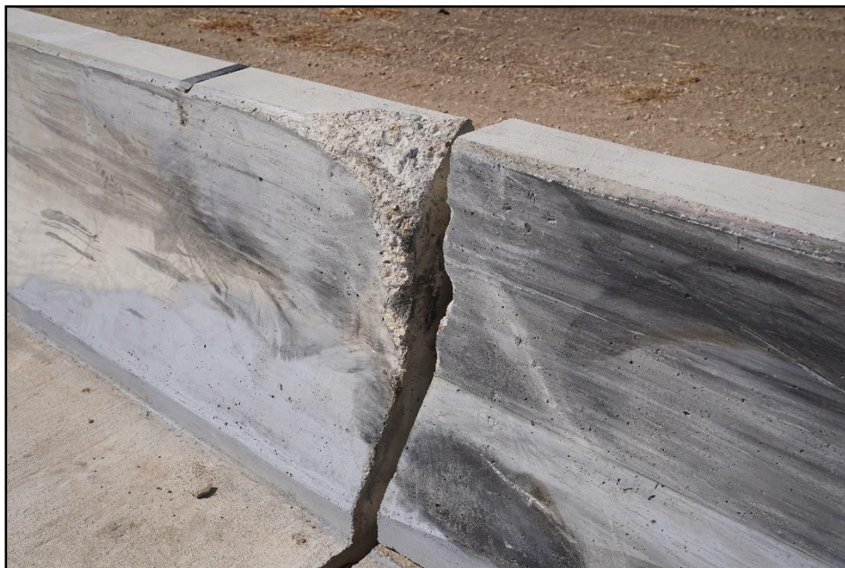
Figure 6.22. Concrete Parapet Shape Transition after Test at the Parapet Joint 611801-03-2.
