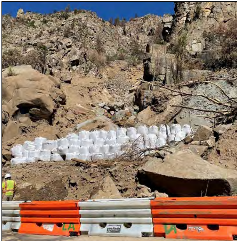
Figure 7.6. Temporary emergency mitigation to prevent further post-wildfire sediment and rock flow onto I-70 in Glenwood Canyon Colorado.
