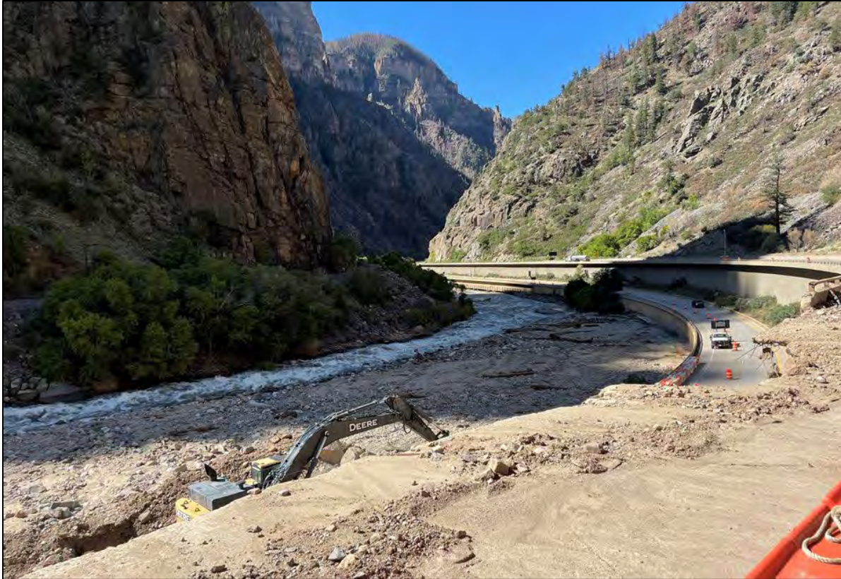
Figure 7.4. Clearing of a post-wildfire debris flow that closed I-70 in Glenwood Canyon, Colorado, in 2021.
