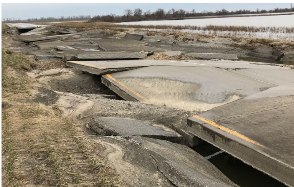
Figure 2: Damaged section of US 34 exhibiting cracked pavement, washed out embankment, and displacement of the roadway. Source: FHWA
