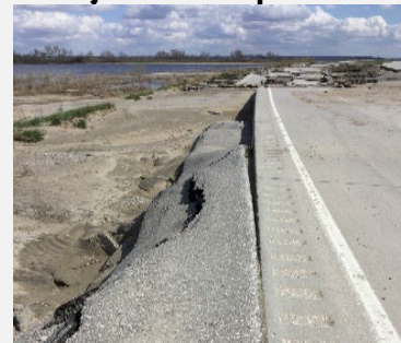
Figure 1: Shows the damage to the roadway embankment and shoulder (US 34). Source: FHWA
