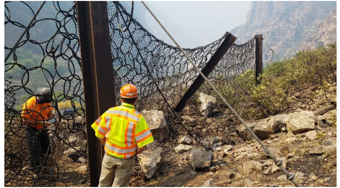
Section of rockfall fencing damaged by a debris flow. Source: FHWA
