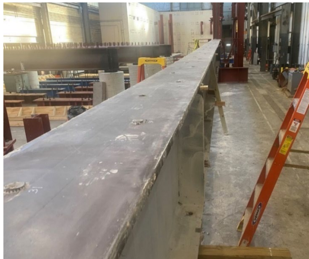
Figure 8.75 – Beam Specimen No. 1 – View of Top Flange for South Half of the Girder After Removal of Concrete Deck
