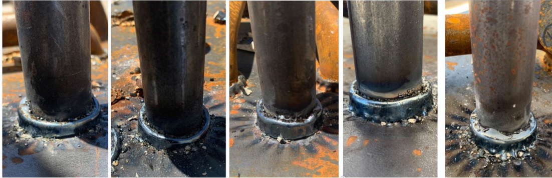
(a) Weld Collar Appearance
