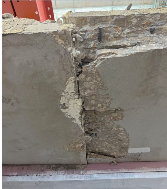
Figure 8.101 – Beam Specimen No. 2 – View Looking Up at the Bottom Side of Deck Showing Crushing at Boundary of PCPs
