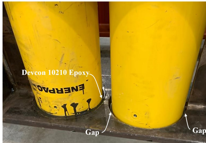
Figure 5.22 - Epoxy is Used to Fill the Gap Between Actuators and Lateral Support
