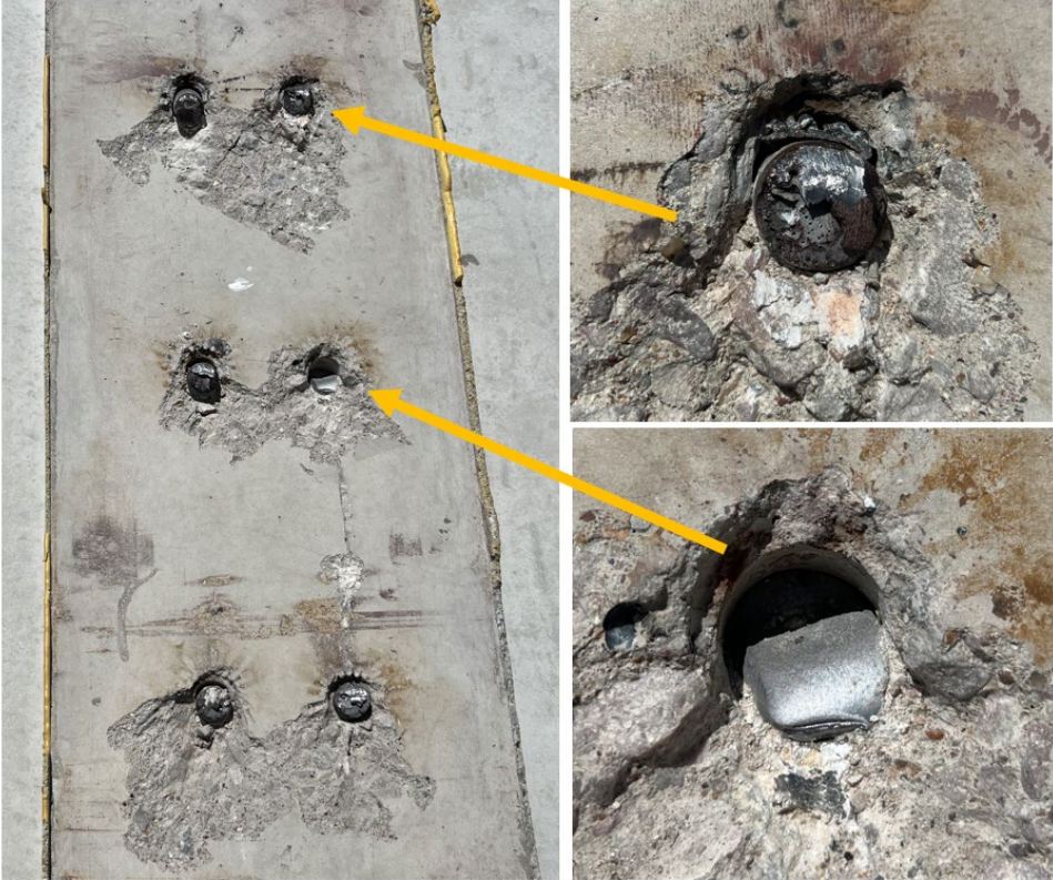
Figure 6.8 - Specimen No.4F: Concrete Deck After Failure with Enlarged Photos of Studs
