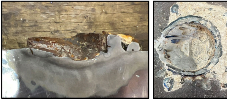
Fracture in the weld or between HAZ and weld 16th stud
