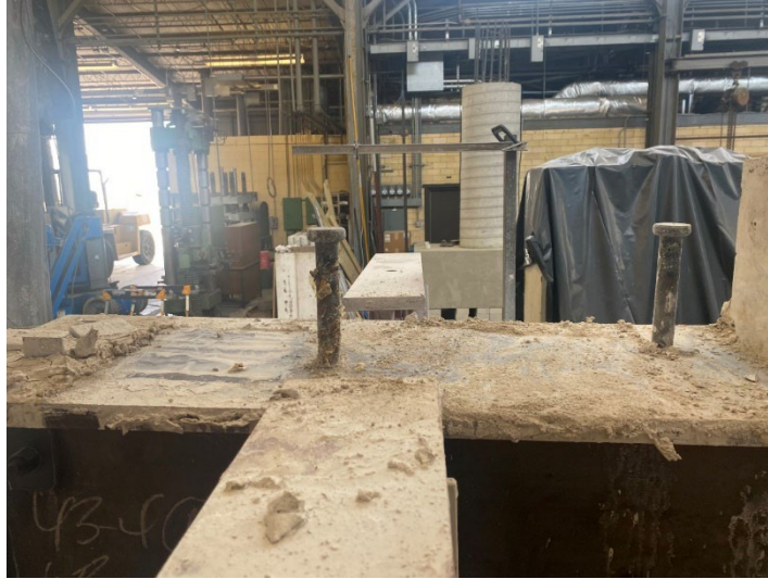
Figure 8.76 – Beam Specimen No. 1 – Shear Studs on North Half of Beam After Removal of Concrete Deck
