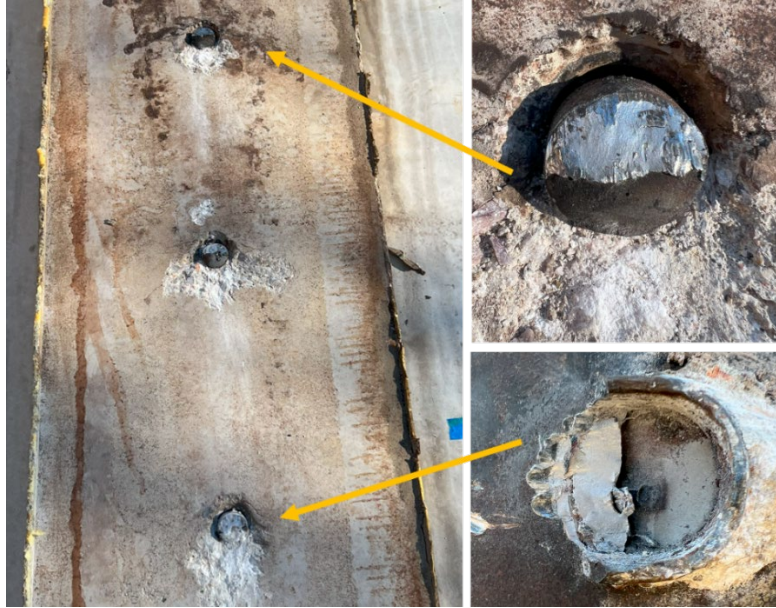
Figure 6.10 - Specimen No.1F: Concrete Deck After Failure Under Monotonic Loading with Enlarged Photos of Studs
