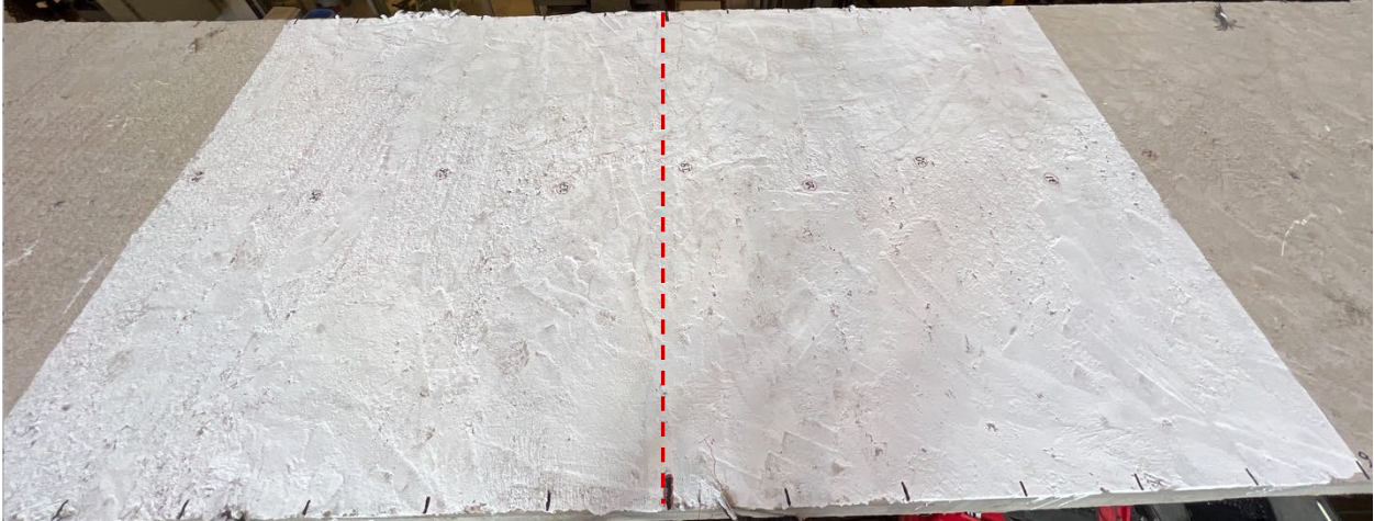
Figure 8.65 – Beam Specimen No. 1 - Portion of Deck over Interior Support Prepared for Tracking Cracks
