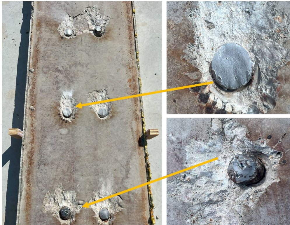
Figure 6.12 - Specimen No.3F: Concrete Deck After Failure with Enlarged Photos of Studs
