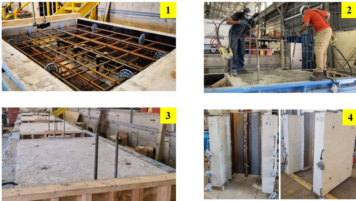
Figure 5.26 - Fabrication Process for Specimen (1) Steel Beam and Reinforcement Placed in the Formwork (2) Concrete Being Cast and Vibrated (3) Concrete Being Cured Inside the Formwork (4) Specimens Removed from the Formwork
