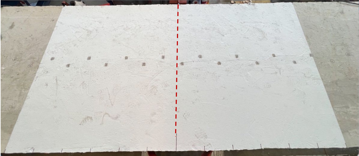
Figure 8.89 - Beam Specimen No. 2 - Portion of Deck over Interior Support Prepared for Tracking Cracks
