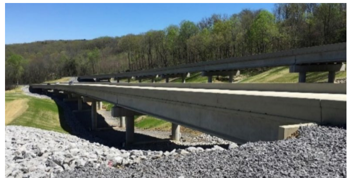
Figure 3: Side view of the completed US 231 bridges illustrating the colluvial deposit and elevation difference of the two roadways. Source: ALDOT
