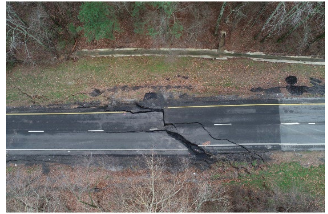
Figure 2: Damage to the southbound lane of US 231 following the February 2020 rainfall event. Source: ALDOT
