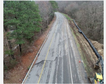
Figure 1: Damage to the northbound lane of US 231 and the berm ALDOT first built along the roadway to minimize further damage and keep water away from the area. Source: ALDOT
