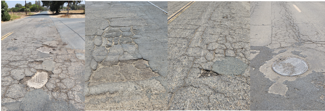
Figure 21. Sample Images of Potholes and a Manhole Cover Gathered with the Visible Light Camera
