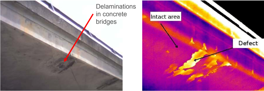
Figure 3. Example Images of a Bridge Taken with a Visible Camera (left) as well as an Infrared Camera (right)
