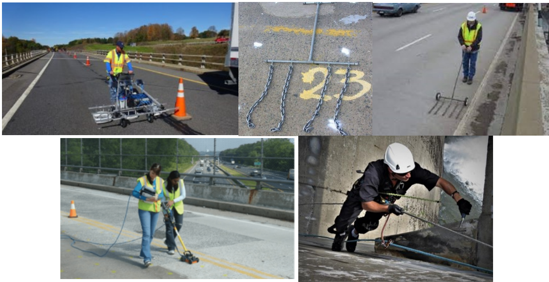
Figure 2. Inspection Methods Used for Bridge and Road Inspection Include Ground Penetrating Radar, a Chain Drag and Other Tools (USDOT-FHWT)
