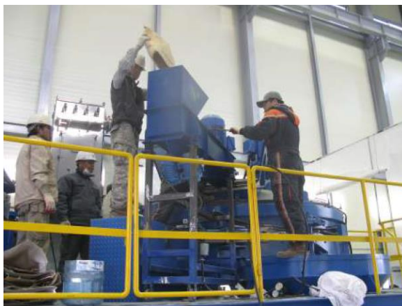
(a) Fiber addition into a feeder
