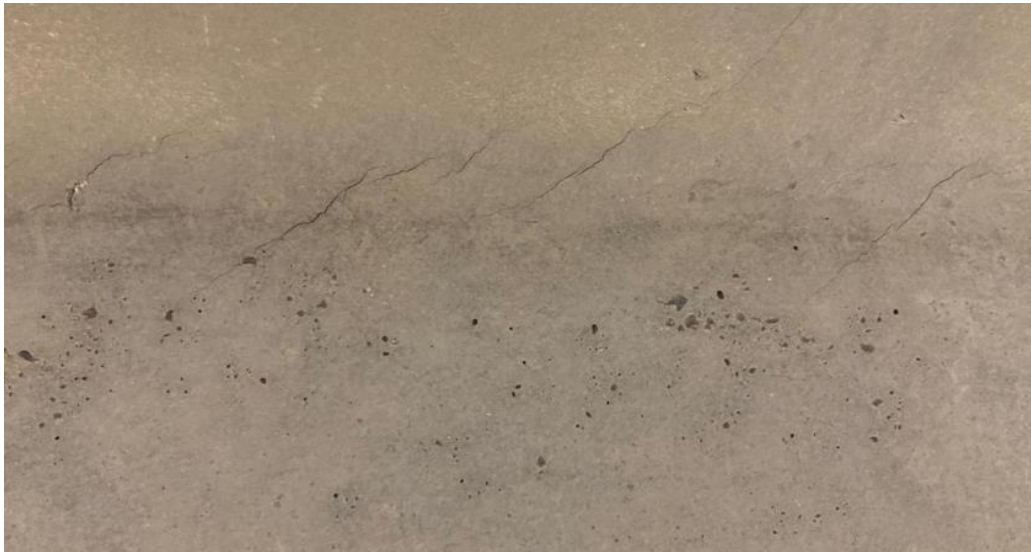
(b) Diagonal Cracks at Junction of Top Flange and Web (3.5 ft to 6.5 ft from East End)
