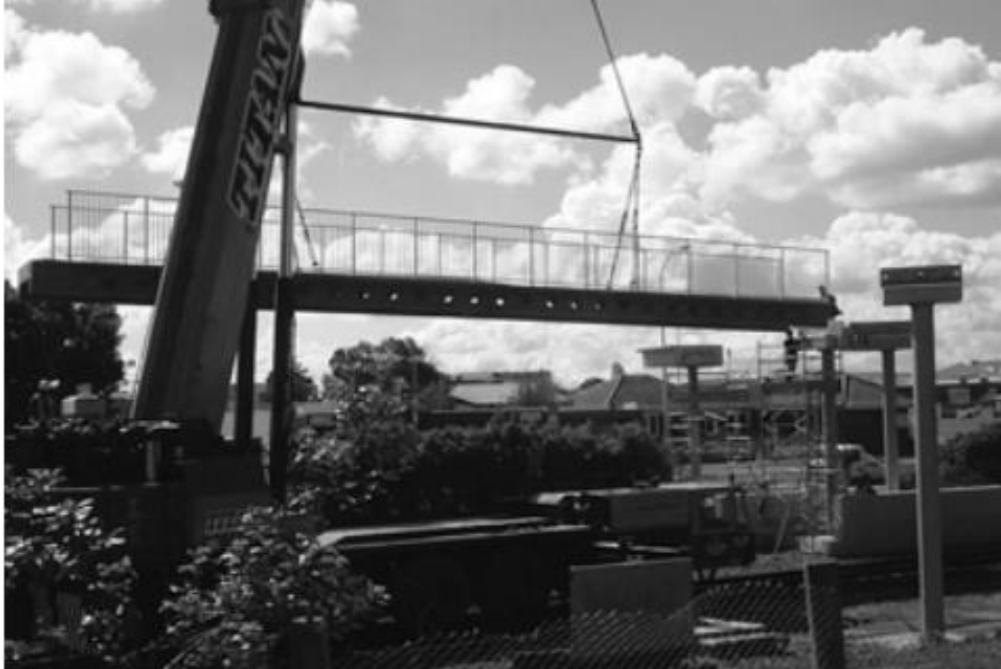
Figure 2.18. Lifting of UHPC Spans with the Railing of Papatoetoe Footbridge, New Zealand (Rebentrost et al. 2008).
