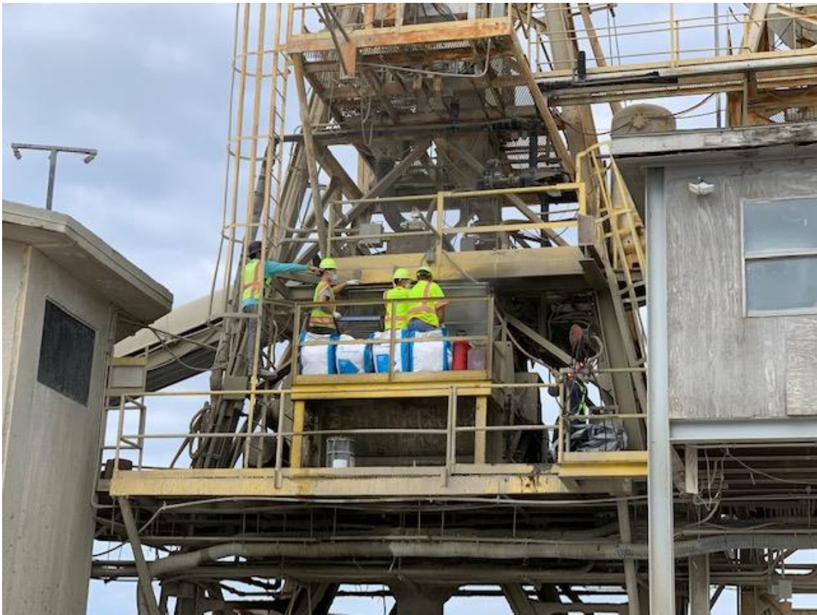
Figure 6.3. Loading Bags of Silica Fume and Steel Fibers on the Mixer Platform.
