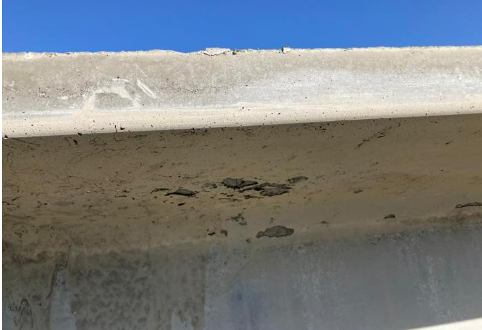
(a) Peeling of UHPC after Removal of Forms at Top Flange
