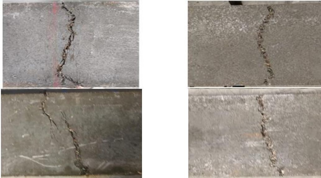
(a) As-cast specimen 01-04: Fibers bridge the crack and result in ductile behavior up to 0.08 in. midspan deflection
