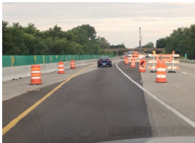
Figure 50. Paint on Lane Shift (FHWA, 2014).
