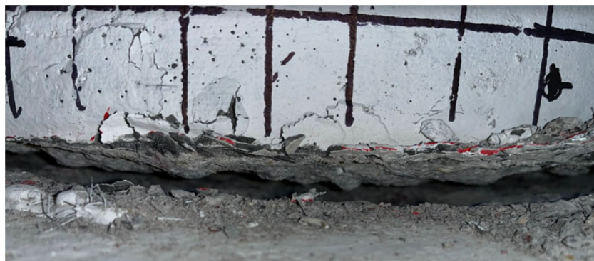
Figure 3.66 Precast 2 Maximum gap Opening at Cycle 18\Delta_y
