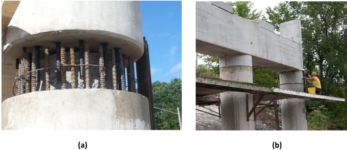
Figure 2.31 (a) Condition of Existing Rebars and New Dowels, (b) Completed Retrofit (Doiron 2016)
