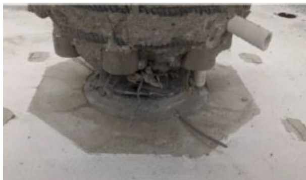
Figure 3.31 Original Precast Bent Pier with Concrete Spalled
