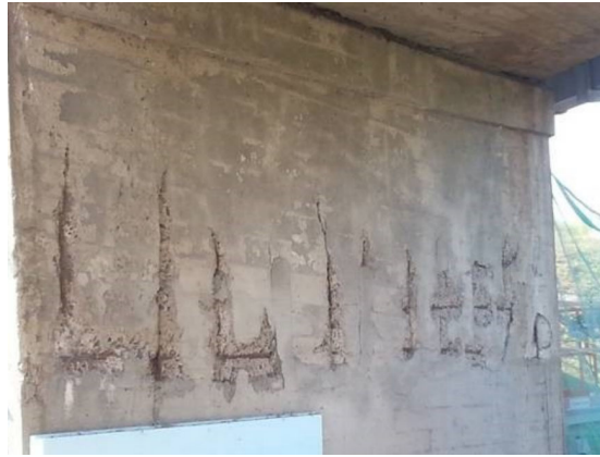
Figure 2.27 Surface of CN Rail Bridge Before Repair ( Doiron 2016 )
