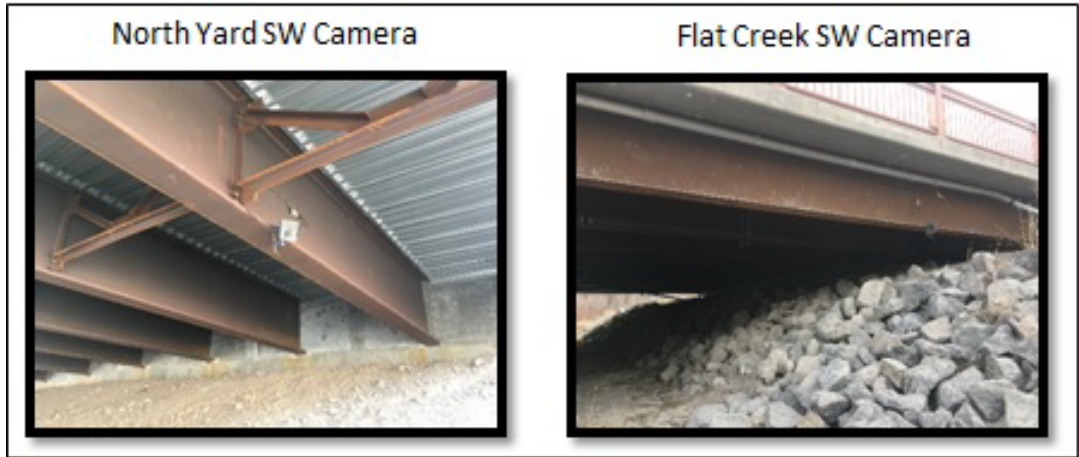
C. Subfigure of photos depicting cameras mounted to bridge girders at North Yard and Flat Creek underpasses.
