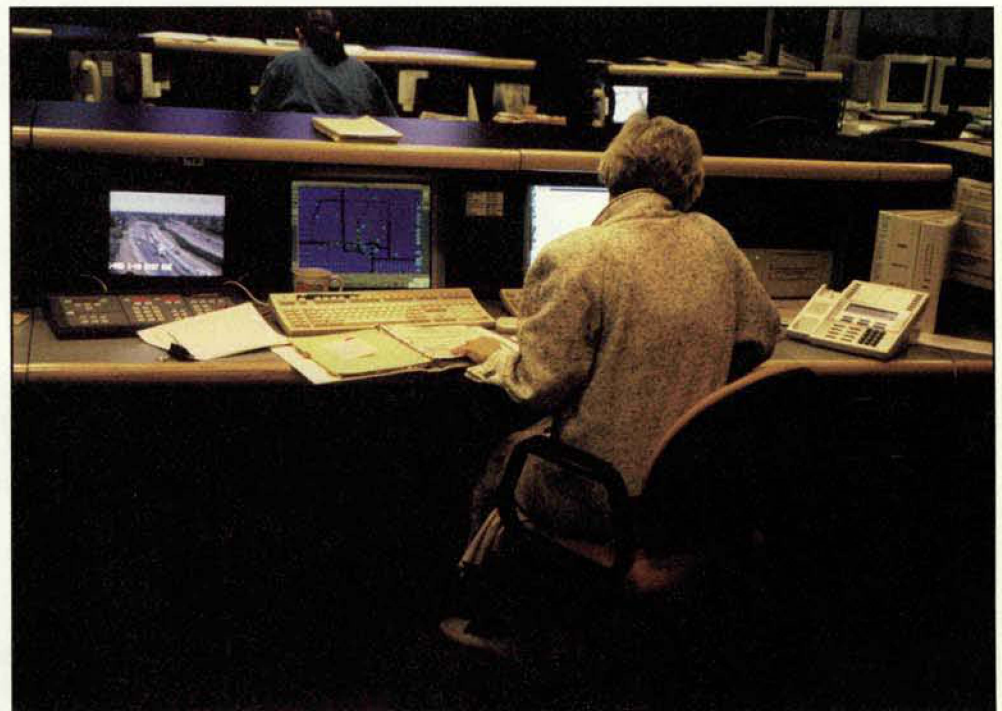
Right: Regional areas across the country are realizing the benefits of having a traffic management system like the one installed in the Phoenix, AZ, metropolitan area. Such systems can manage transit and freeway traffic, provide regional, multimodal traveler information, manage electronic toll collection and incident occurrence and monitor and manage traffic signal control and emergency management services.
