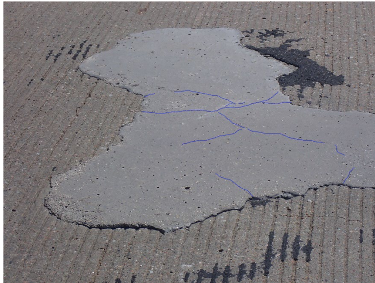
Figure Chapter 4.9 Highlighted cracks on one of the repair patches
