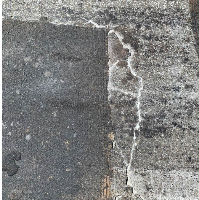
Figure Chapter 2.2 Early minor halo efflorescence on NDOT bridge polymer concrete repair
