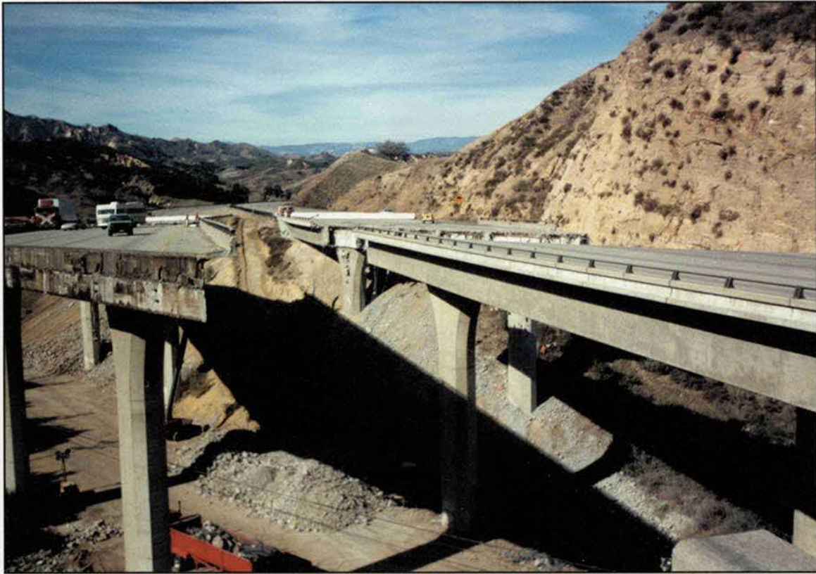
The Los Angeles area also experienced an earthquake in 1993 that sliced I-5 in half along with major damage to other area highways and bridges. A team of seismological experts from FHWA and CALTRANS was on the scene in a matter of hours.
