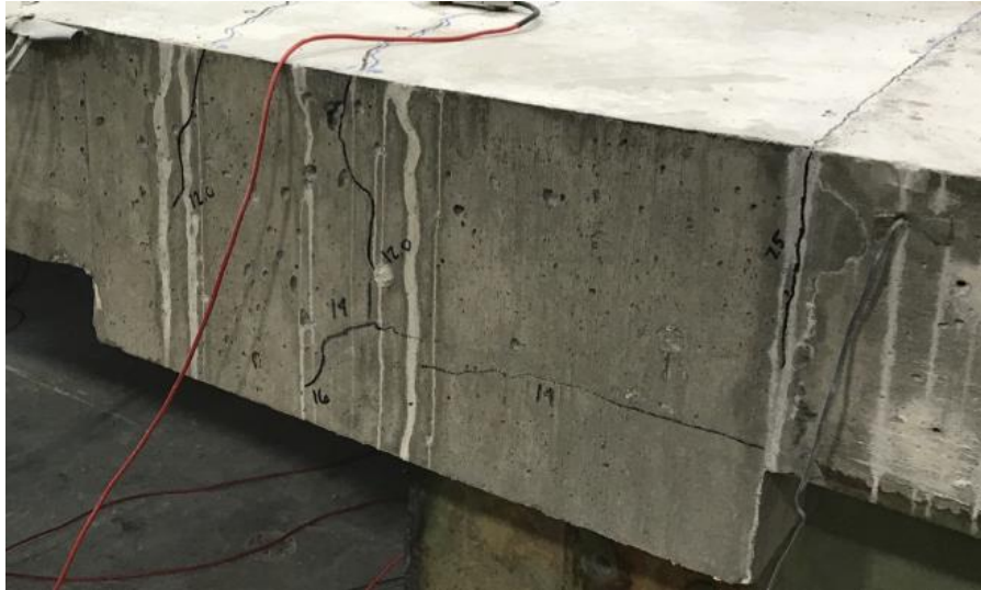
Figure 4.16. Cracking occurring in the concrete diaphragm section at the intersection with the steel girder, Test 1
