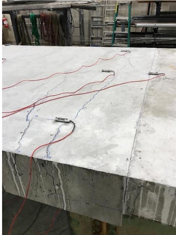
Figure 4.12. Cracking at the construction joint
