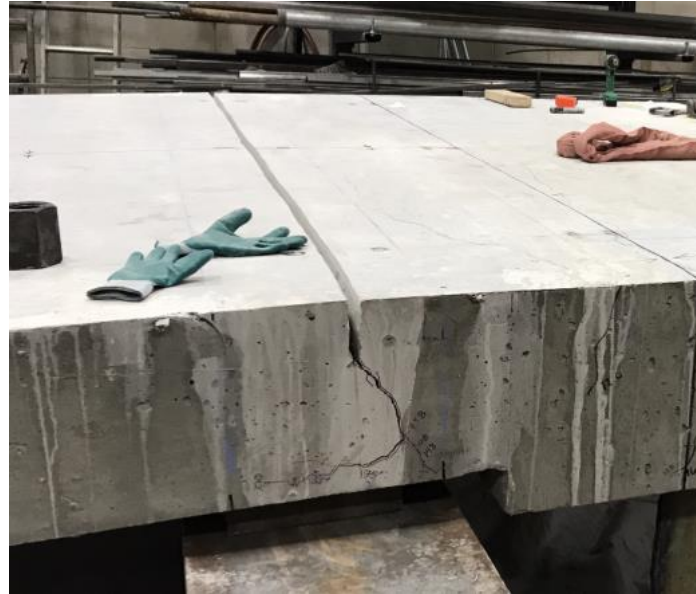
Figure 4.26. Saw cut at the top of the approach slab through the top reinforcing in preparation for Test 2
