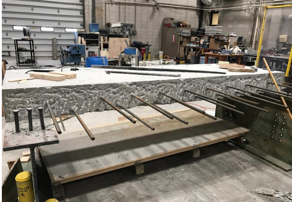
Figure 4.3. Construction joint at interface of existing bridge deck and concrete diaphragm sections
