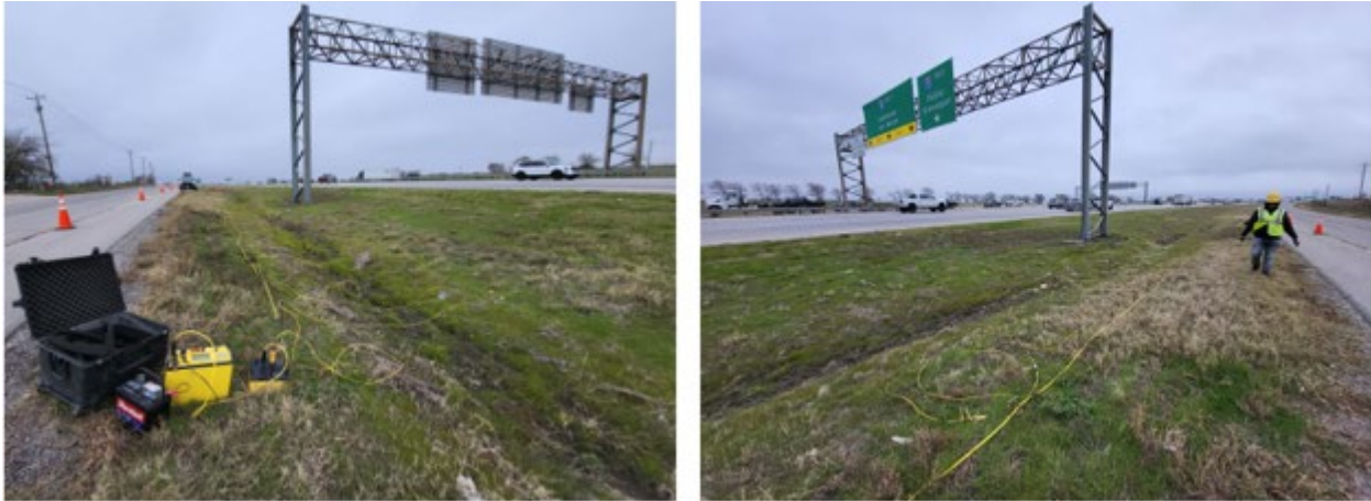
Figure 2.48. Implementation of the ERI along IH 20 at the east side of Farmer Rd
