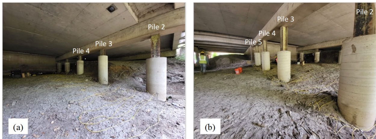
Figure 2.52. Implementation of ERI for SH 352 at White Rock Creek; (a) Line 1, (b) Line 2.
