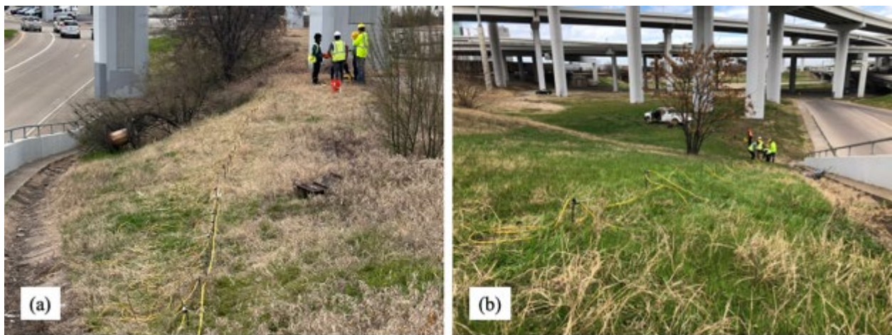
Figure 4.11. Implementation of the ERI at IH 35W and railroad; (a) Line 1 and (b) Line 3
