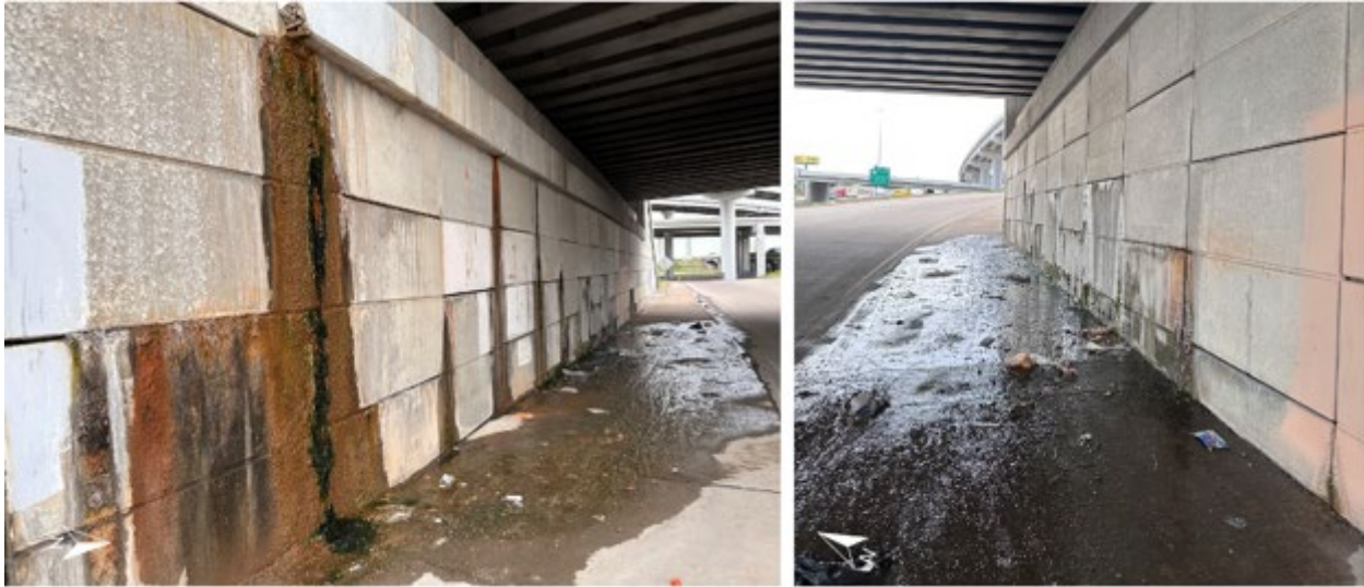
Figure 4.9. Conditions of the retaining wall beneath the bridge at the time of surveying
