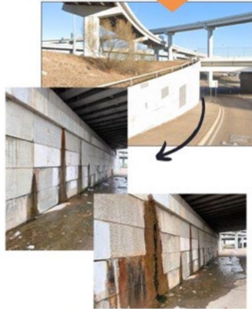
Drainage problem behind the wall.
