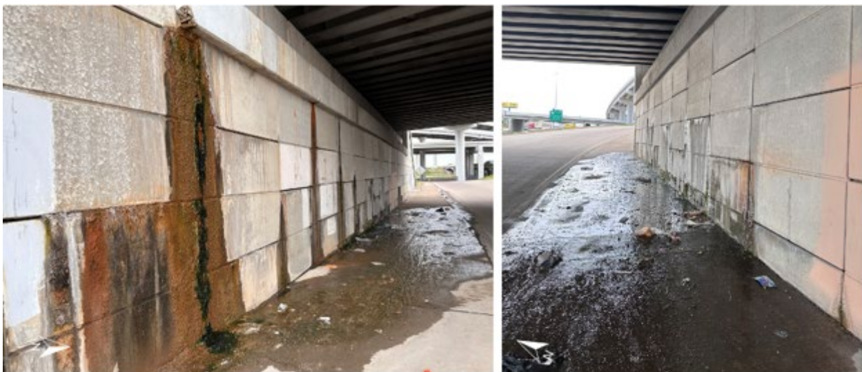
Figure 2.67. Current conditions of the retaining wall beneath the bridge
