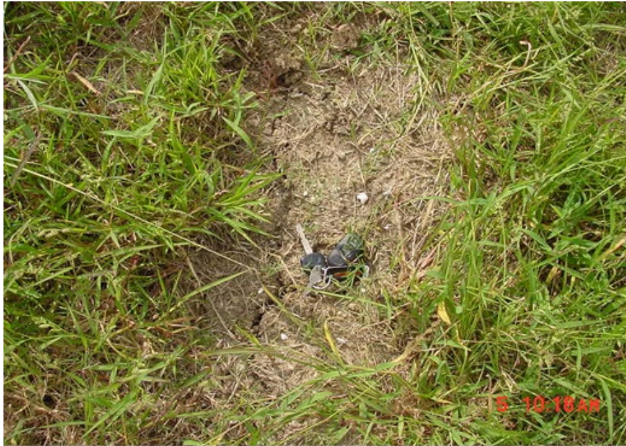
Figure 1. Cracks due to shrinkage of clayey soils along the side of highway embankment
