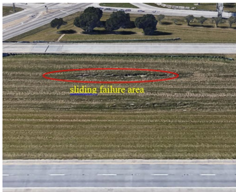
Figure 17. A close view of sliding failure area
